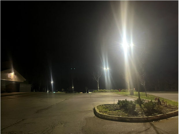
Existing lighting Mountain View Middle School
