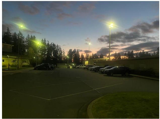
Existing parking lot lighting
