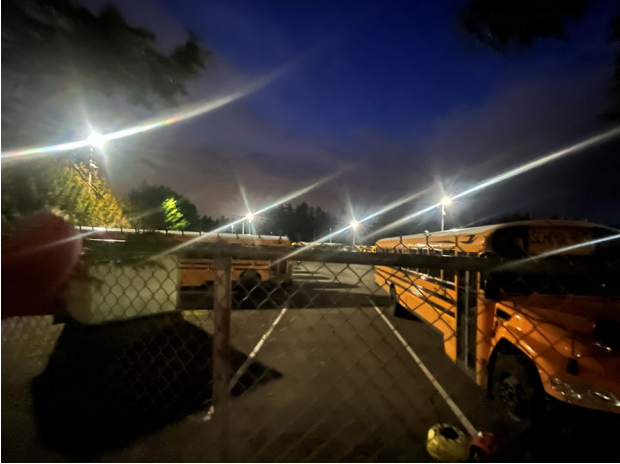
Existing lighting School District Maintenance Facility
