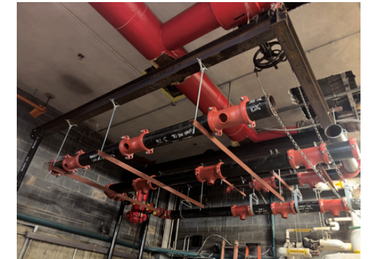
MS Boiler Room Piping + Boiler Pads
