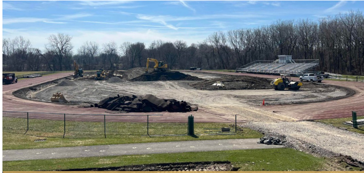
Field has been demolished. Site is being prepped for new turf field.
