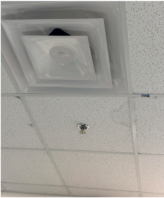
Evidence of moisture damage
