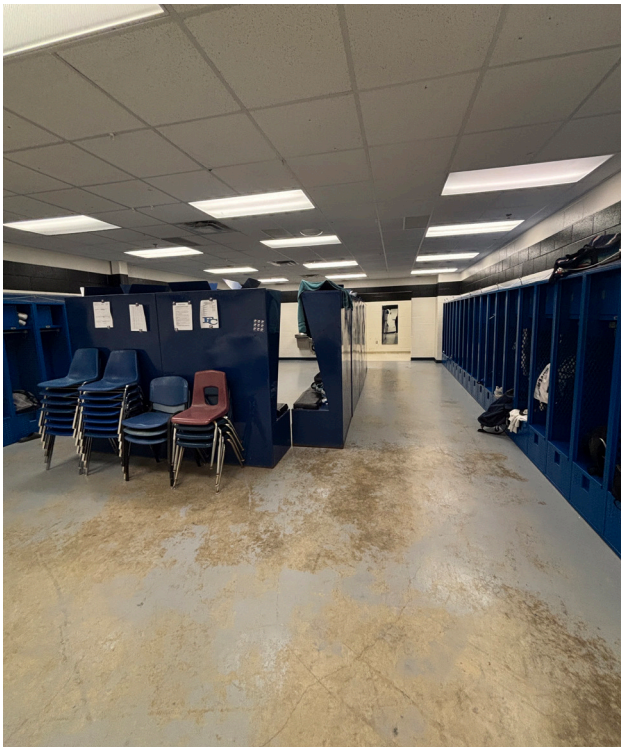
Deteriorating floor finish
