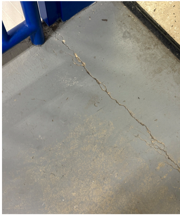
Evidence of structural movement
