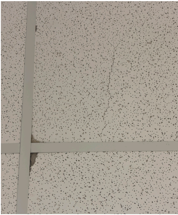
Damaged ceiling tile
