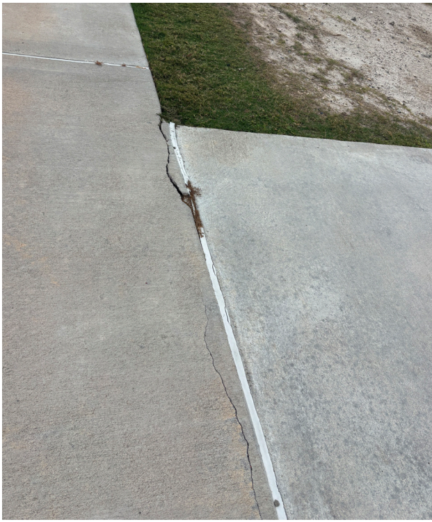
Evidence of structural movement
