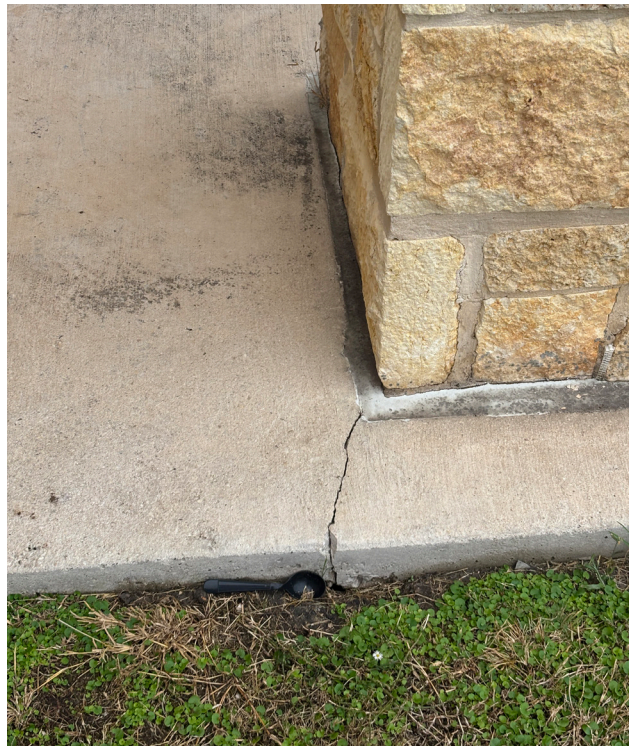
Evidence of structural movement
