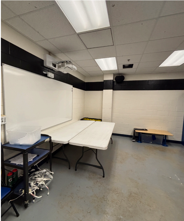
Defective intercom system
