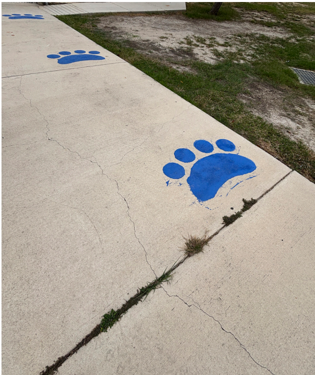
Evidence of structural movement
