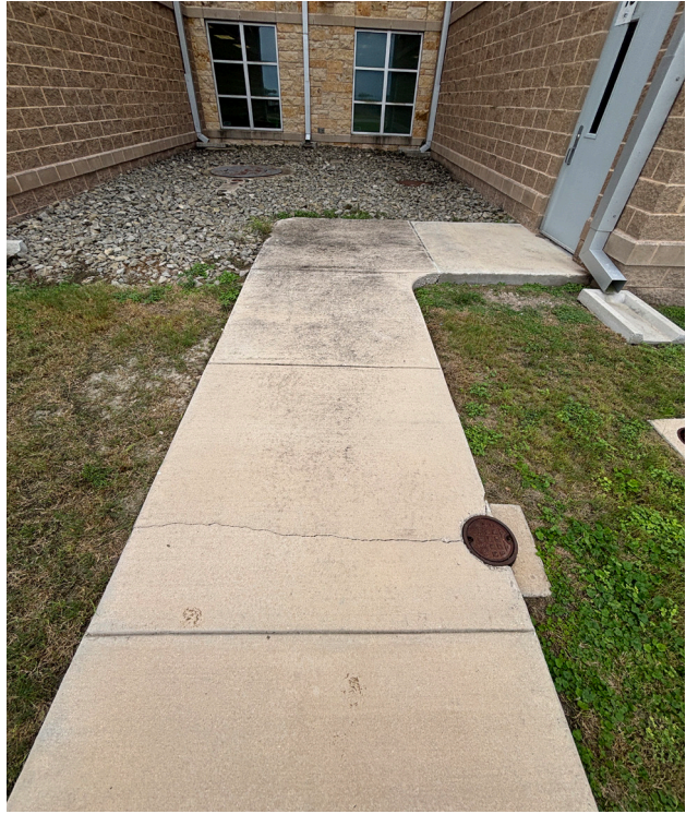
Evidence of structural movement
