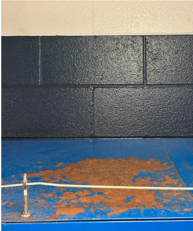
Deteriorating locker finish
