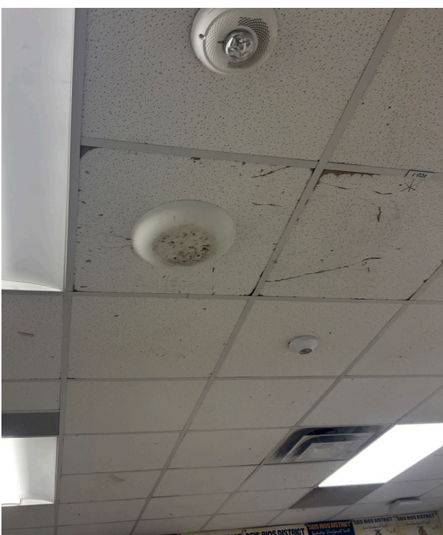
Damaged ceiling tiles
