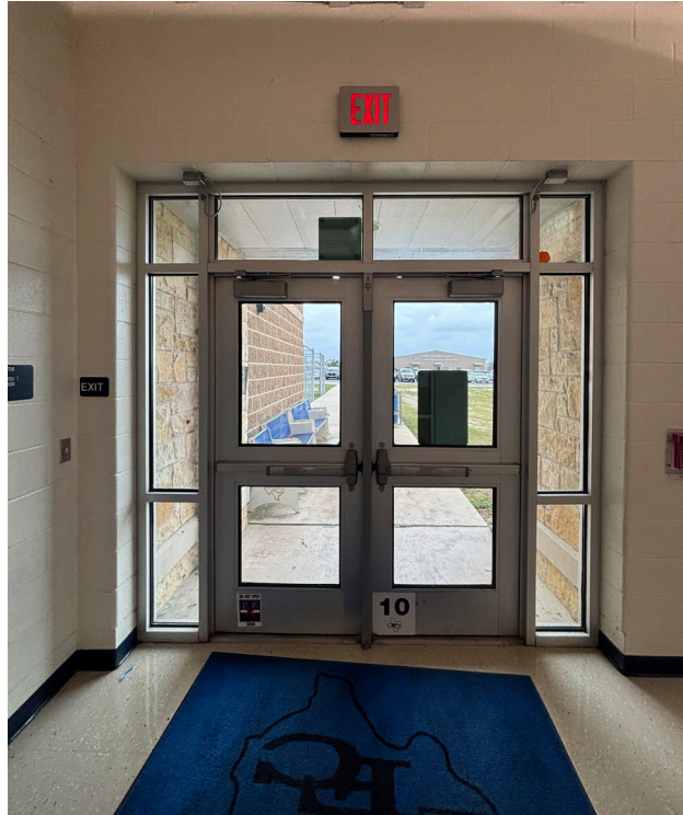
No secure vestibule on 1st floor
