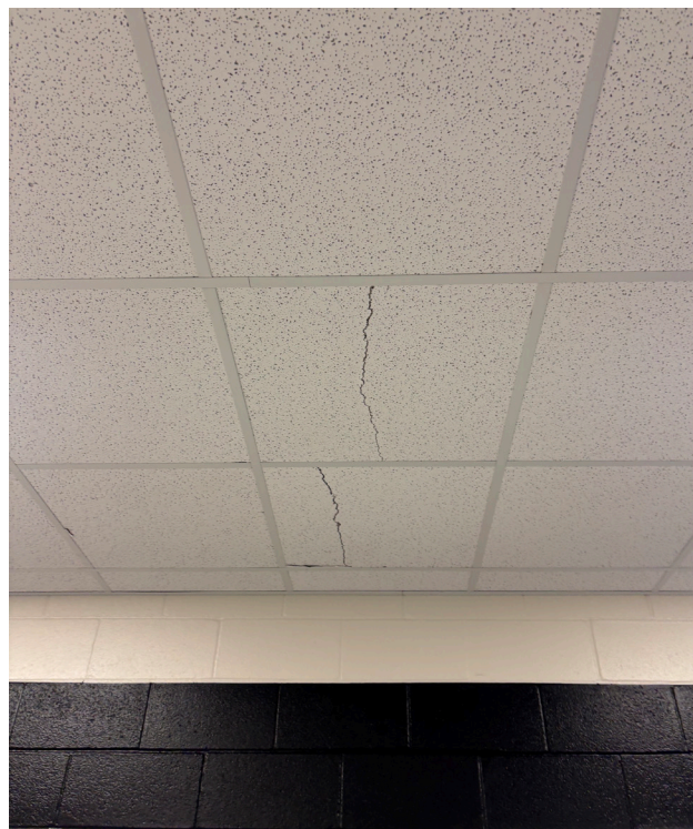
Damaged ceiling tiles
