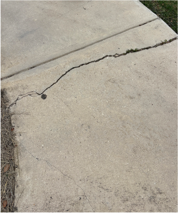
Evidence of structural movement
