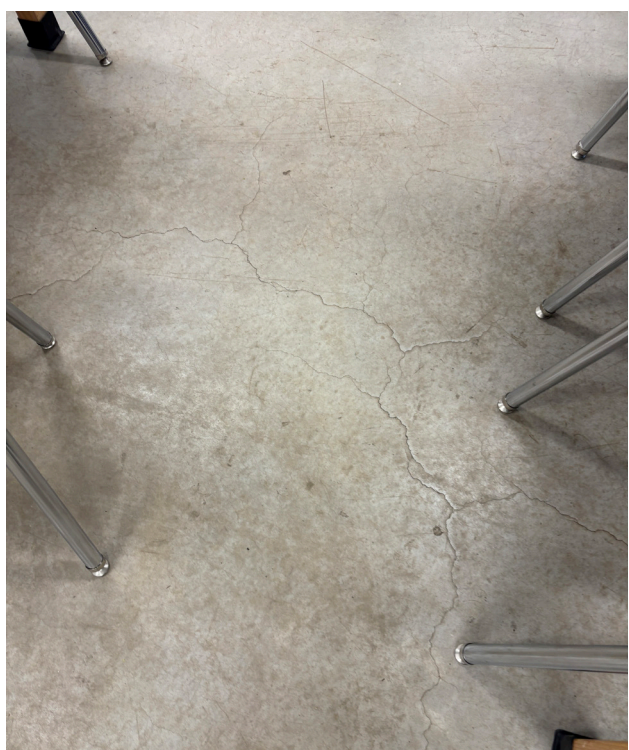
Evidence of structural movement
