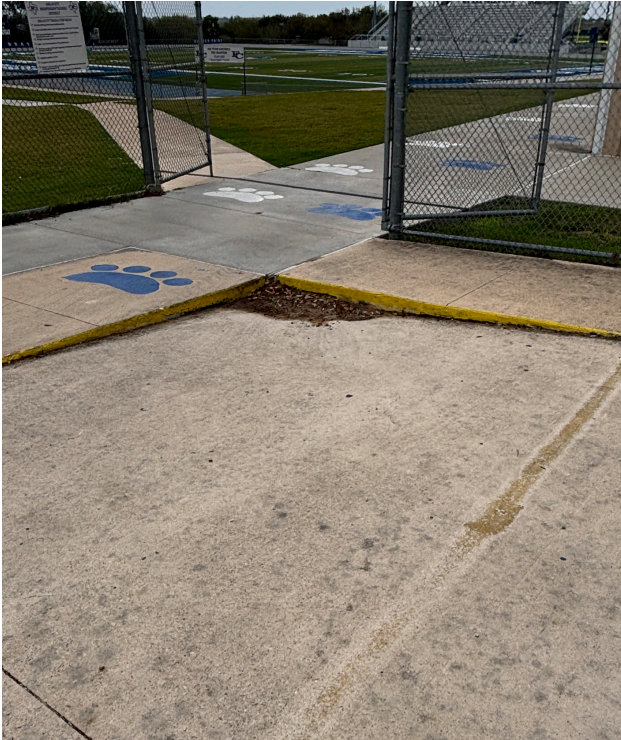
Evidence of structural movement
