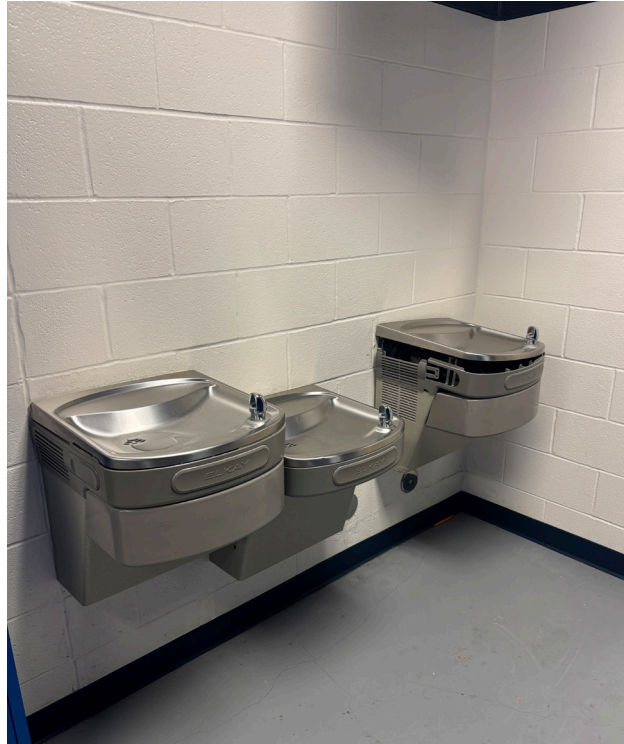
Damaged water fountain
