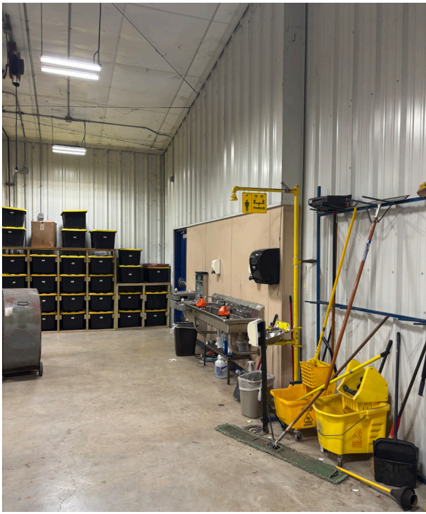
Missing drain at shower
