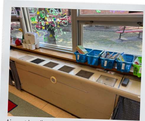
Air vent handlers in Kensington classrooms are approximately 60 years old, and would be replaced along with their connected shelving units.
