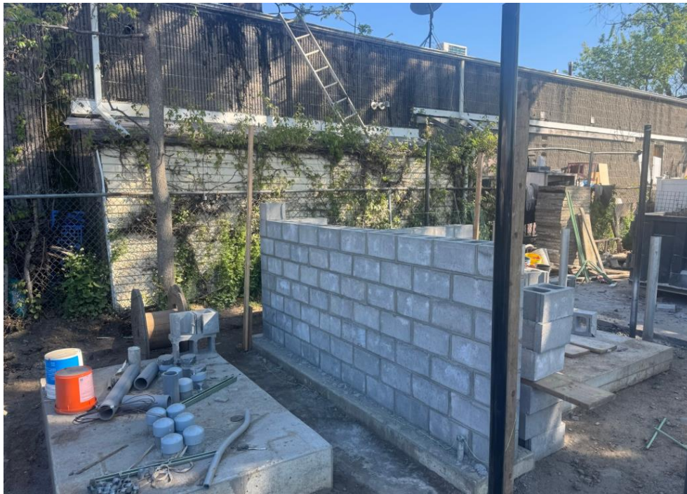
Hempstead IAQ – Paterson Transformer Pad
