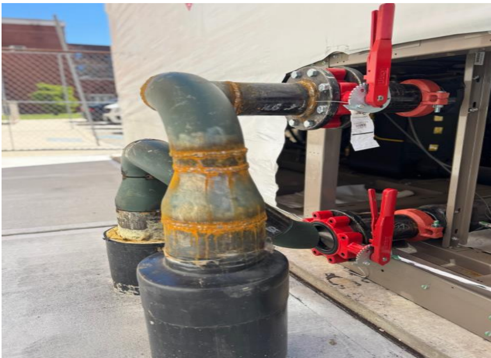
Hempstead IAQ – Prospect ES CHW Piping
