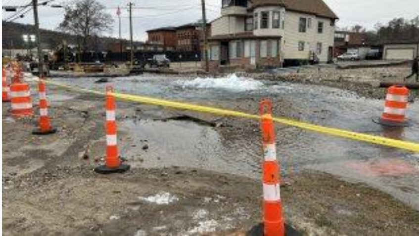
WATER MAIN BREAK IMPACTS SCHOOLS One side of Sprague Elementary School (brick building above) on 1443 Thomaston Avenue in Waterbury, Conn. can be seen along with water gushing from the water main break as of Saturday, Dec. 13, 2025, causing school closures Monday-Wednesday, Dec. 15-17. Photo from NBC CT News
