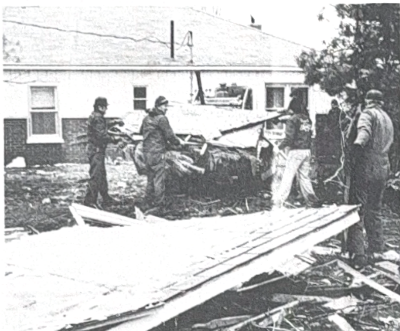
With the help of a bulldozer, neighbors Saturday afternoon clear off debris from the George Szymkowski home, 6845W County Road 450N, where the tornado lifted off the roof of the garage and family room. (News-Dispatch photo by Bill Swedenberg)
