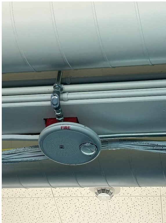
Sensor bound into plenum of cables
