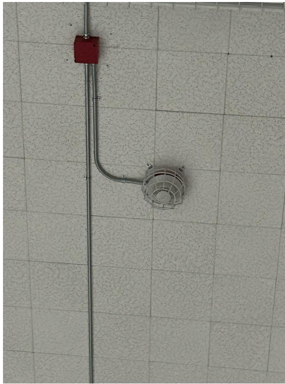
Higher reach tile similar to lower levels tile
