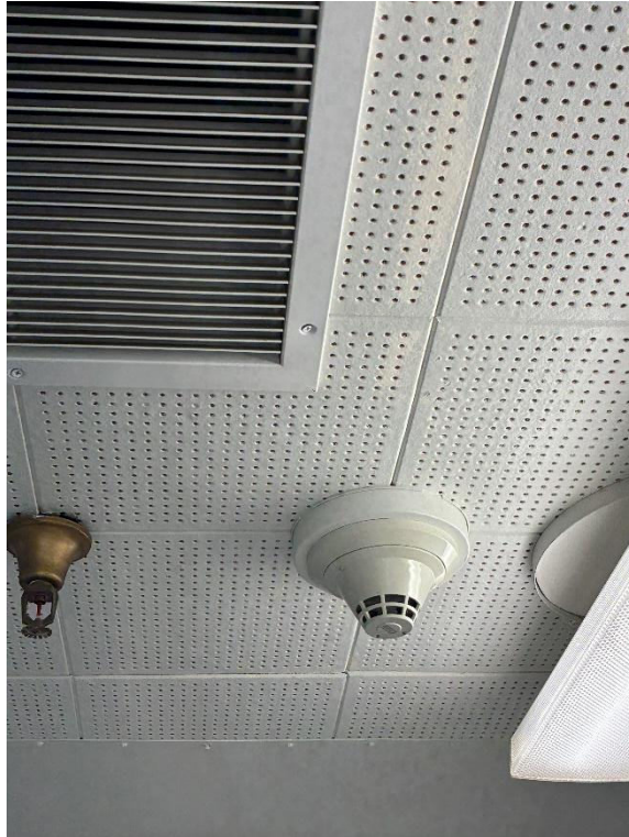
Close up of fire sensor
