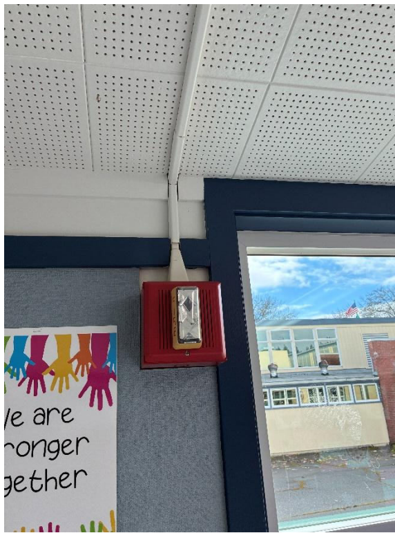
Fire alarm – typical wall mount
