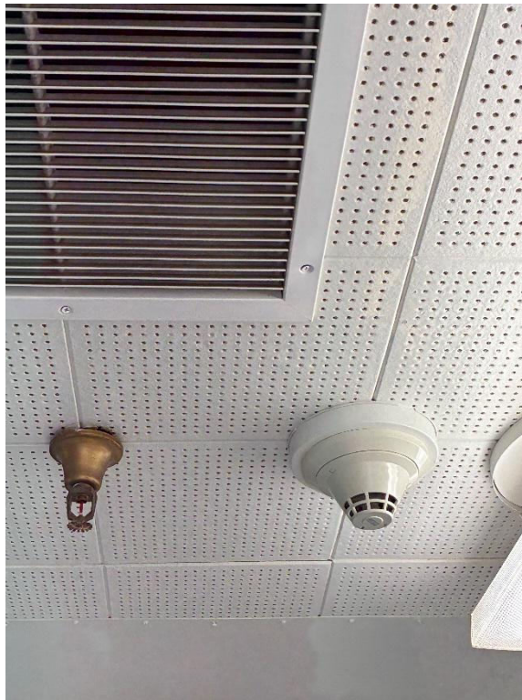
Fire suppression system and sensor
