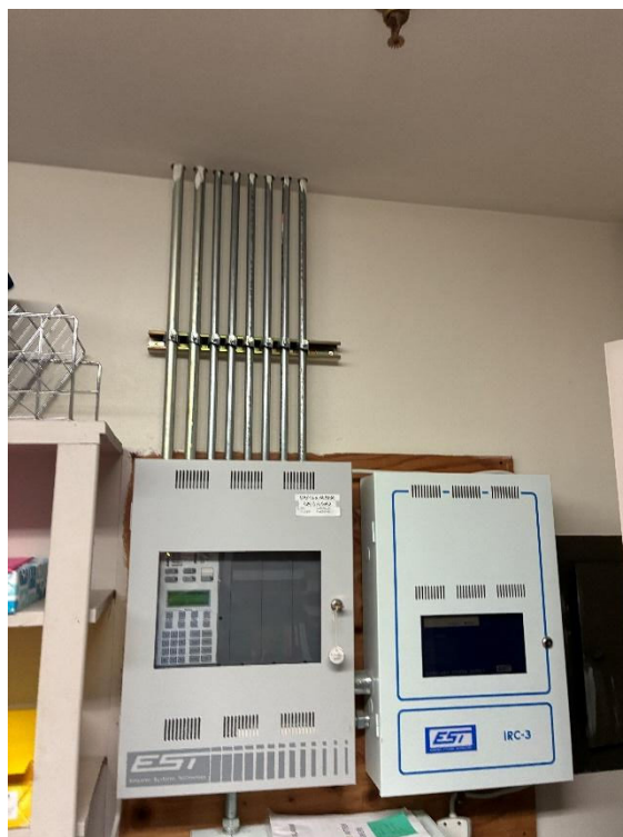
Fire system controller
