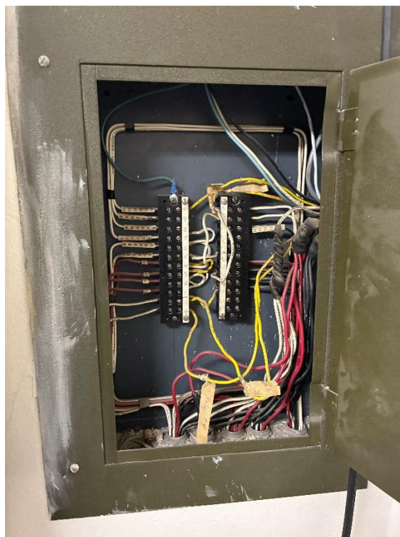
Older wiring system
