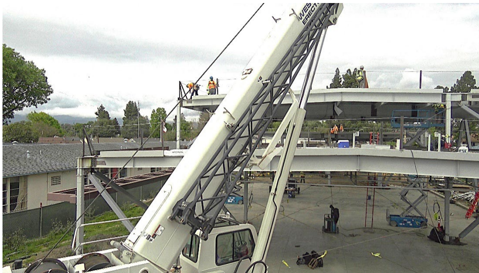
Views from the webcam in the rear playground looking toward the front parking lot. April 1, 2026 This view highlights the difficulty in coordinating construction and school activities.
