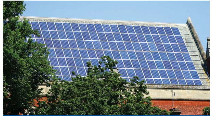
Roof-mounted solar panels
