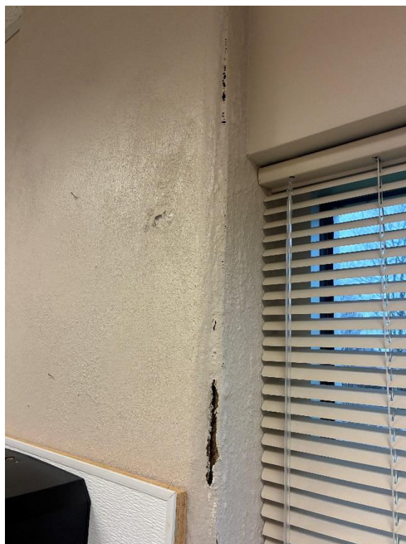
Water impacted beam interior
