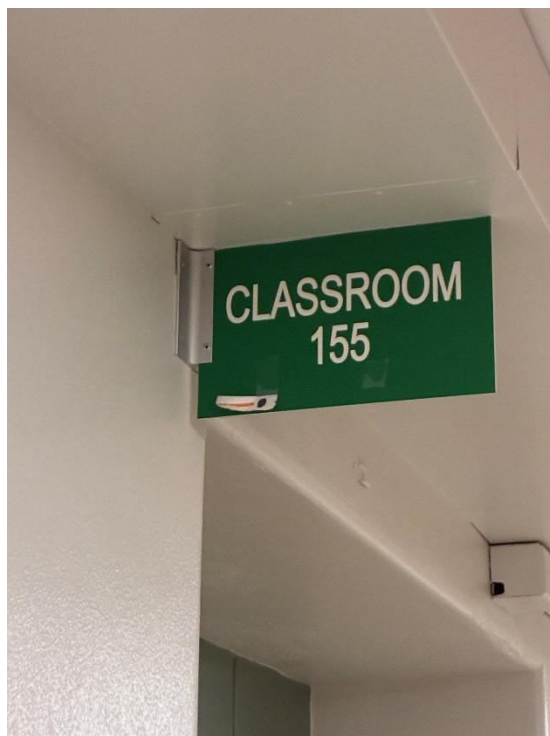
Classroom impacted by exterior wall
