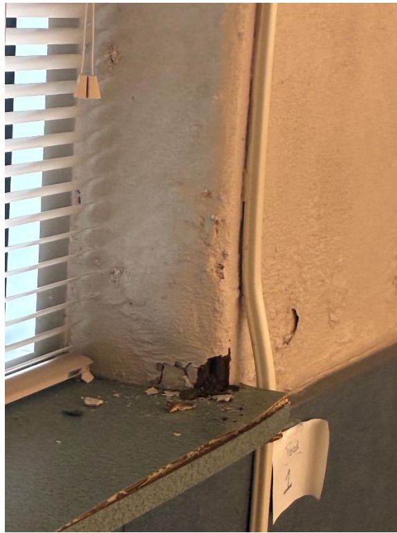
Plaster decay onto sill
