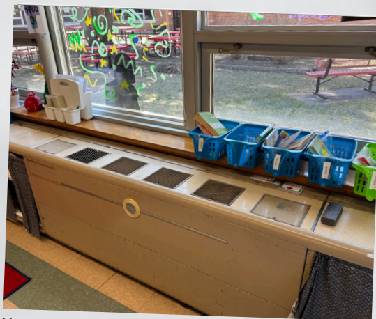
Air vent handlers in Kensington classrooms are approximately 60 years old, and would be replaced along with their connected shelving units.
