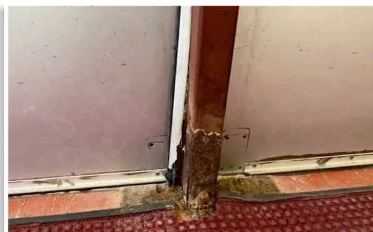
Much of the proposal renovates structures in the Middle School, such as these doors that have rusted out at their base.
