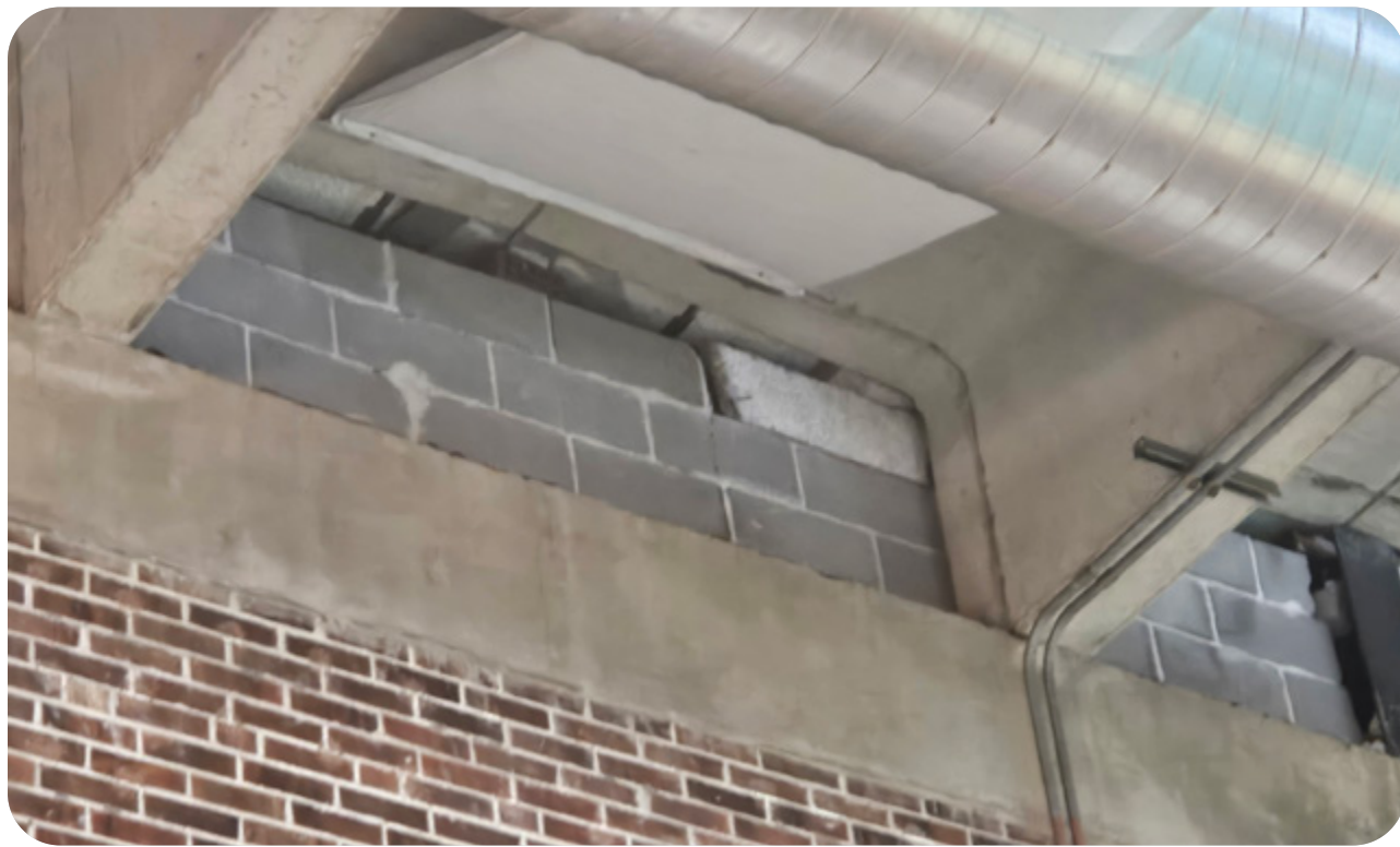
Failing indoor masonry at pool
