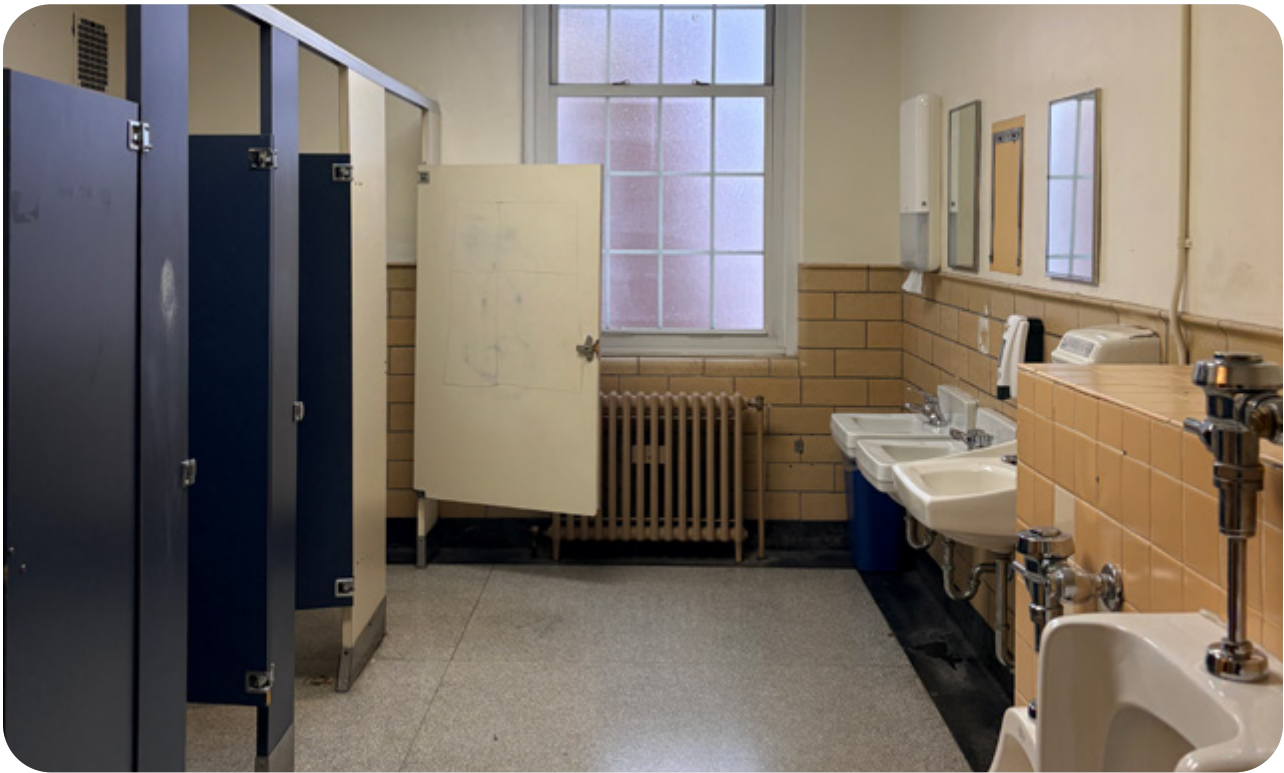
Needed toilet room upgrades
