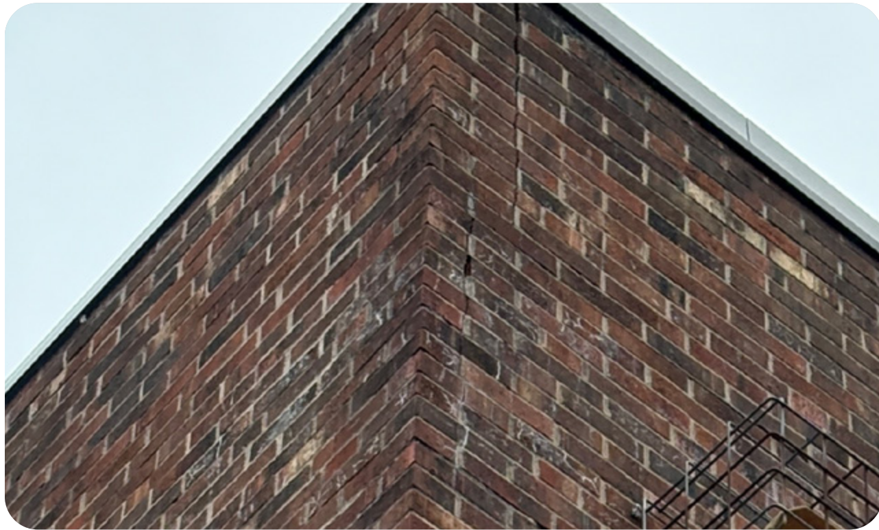
Failing exterior masonry at pool
