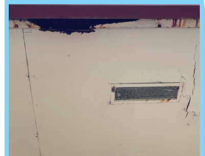
DETERIORATING ROOF AT ELKHORN ELEMENTARY.
