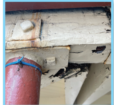
DRY ROT WOOD BEAMS AT PRUNEDALE ELEMENTARY SCHOOL.
