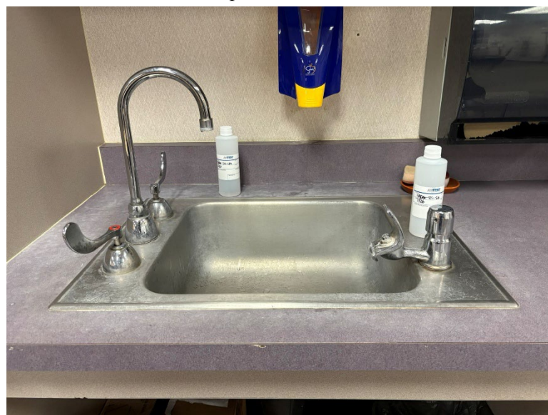
Room 114 Tap – Sample 31126-SIS-49 Room 114 Fountain – Sample 31126-SIS-50
