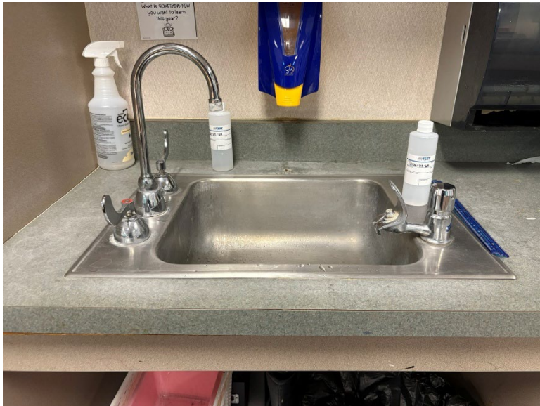
Room 307 Tap – Sample 31126-SIS-67 Room 307 Fountain – Sample 31126-SIS-68
