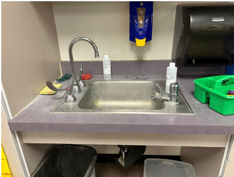
Room 105 Tap – Sample 31126-SIS-28 Room 105 Fountain – Sample 31126-SIS-29
