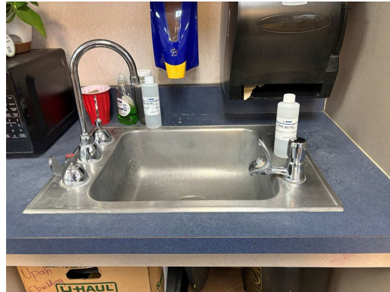
Room 203 Tap – Sample 31126-SIS-91 Room 203 Fountain – Sample 31126-SIS-92
