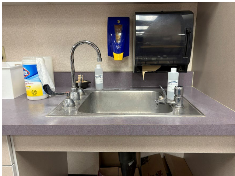
Room 111 Tap – Sample 31126-SIS-43 Room 111 Fountain – Sample 31126-SIS-44
