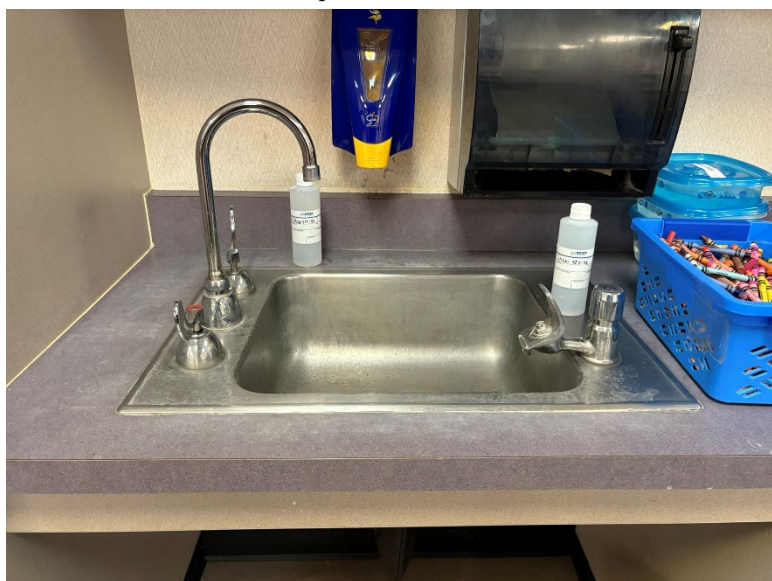
Room 113 Tap – Sample 31126-SIS-47 Room 113 Fountain – Sample 31126-SIS-48
