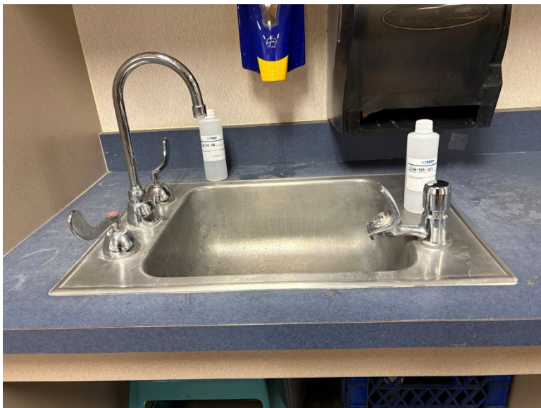
Room 207 Tap – Sample 31126-SIS-106 Room 207 Fountain – Sample 31126-SIS-107
