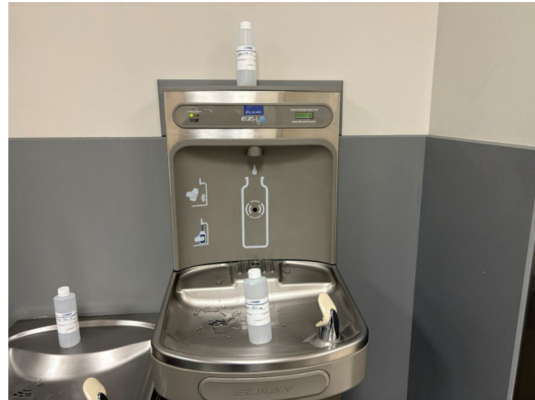
Outside Office Right Fountain – Sample 31126-SIS-12 Outside Office Bottle Filler – Sample 31126-SIS-13
