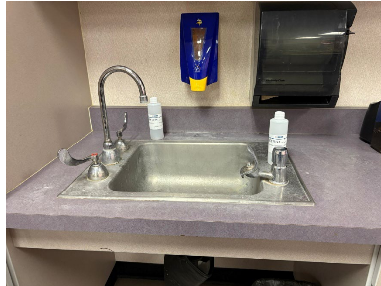
Room 105 Tap – Sample 31126-SIS-26 Room 105 Fountain – Sample 31126-SIS-27
