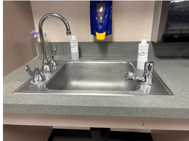
Room 311 Tap – Sample 31126-SIS-61 Room 311 Fountain – Sample 31126-SIS-62
