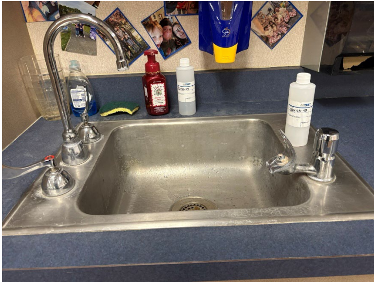
Room 206 Tap – Sample 31126-SIS-97 Room 206 Fountain – Sample 31126-SIS-98
