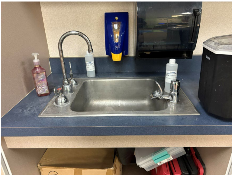
Room 211 Tap – Sample 31126-SIS-114 Room 211 Fountain – Sample 31126-SIS-115
