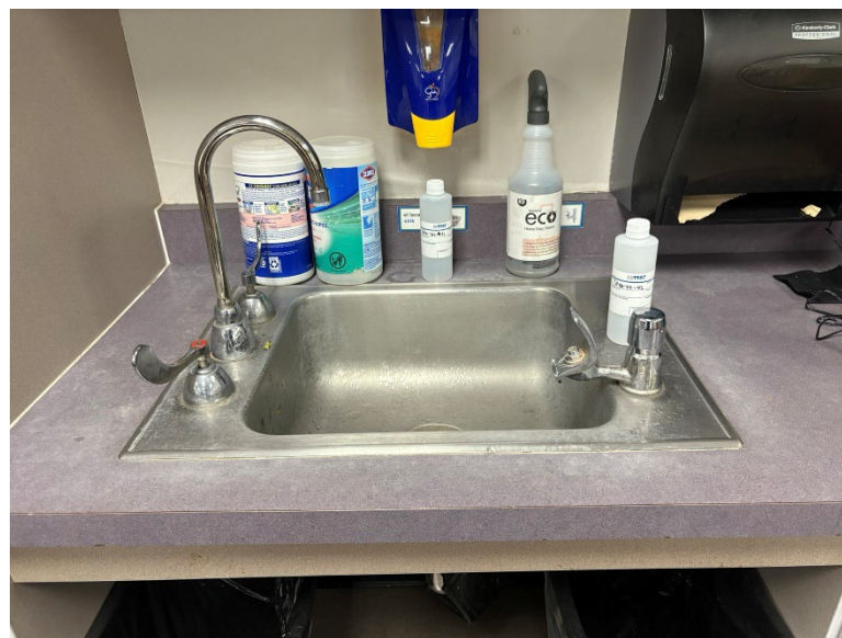
Room 110 Tap – Sample 31126-SIS-41 Room 110 Fountain – Sample 31126-SIS-42
