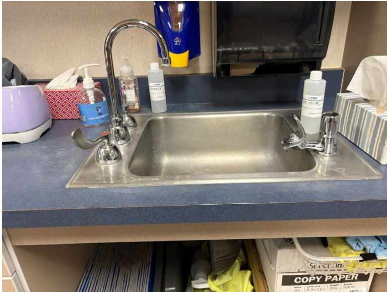
Room 213 Tap – Sample 31126-SIS-118 Room 213 Fountain – Sample 31126-SIS-119
