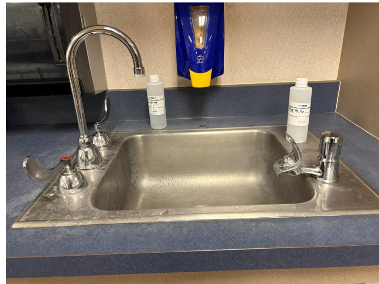
Room 205 Tap – Sample 31126-SIS-95 Room 205 Fountain – Sample 31126-SIS-96
