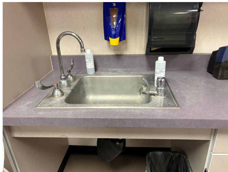
Room 102 Tap 1 – Sample 31126-SIS-19 Room 102 Fountain – Sample 31126-SIS-20
