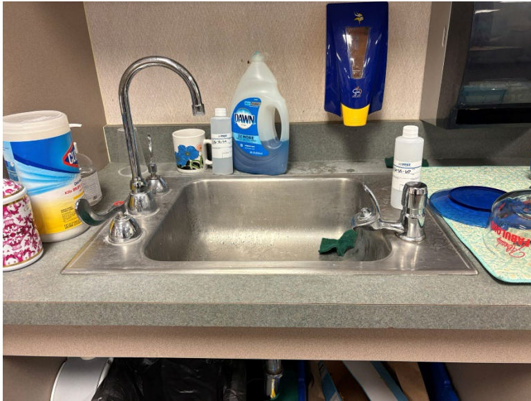
Room 312 Tap – Sample 31126-SIS-59 Room 312 Fountain – Sample 31126-SIS-60
