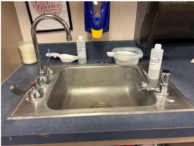
Room 204 Tap – Sample 31126-SIS-93 Room 204 Fountain – Sample 31126-SIS-94
