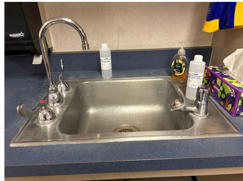
Room 210 Tap – Sample 31126-SIS-108 Room 210 Fountain – Sample 31126-SIS-109
