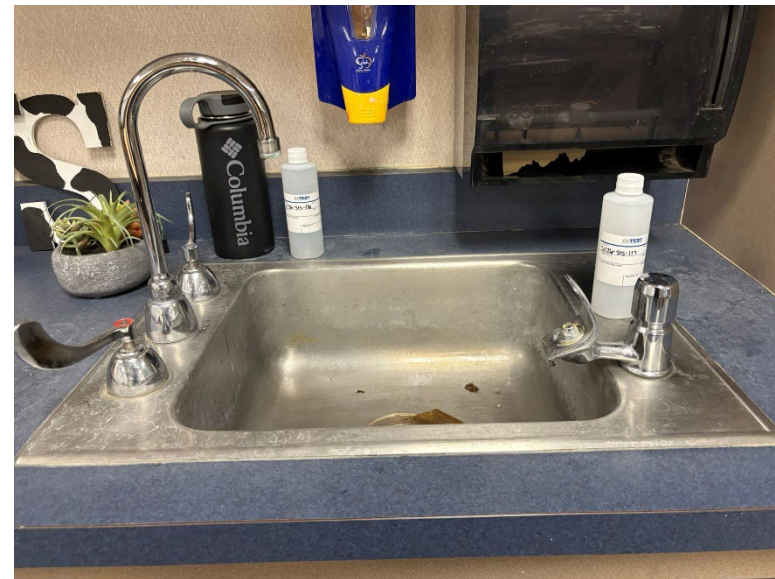
Room 214 Tap – Sample 31126-SIS-116 Room 214 Fountain – Sample 31126-SIS-117
