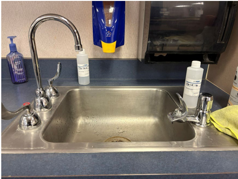
Room 202 Tap – Sample 31126-SIS-89 Room 202 Fountain – Sample 31126-SIS-90
