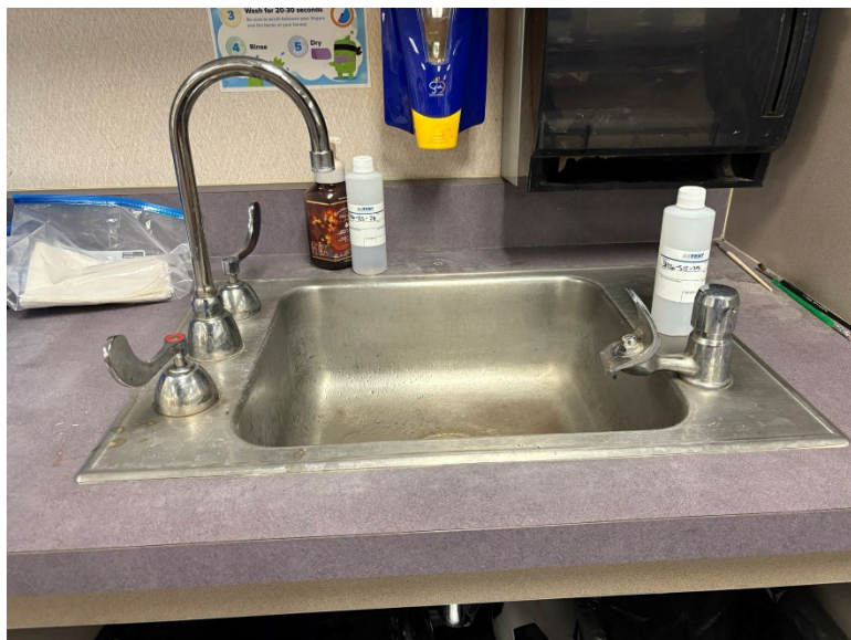
Room 101 Tap – Sample 31126-SIS-17 Room 101 Fountain – Sample 31126-SIS-18
