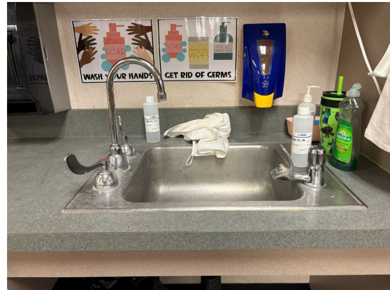
Room 314 Tap – Sample 31126-SIS-57 Room 314 Fountain – Sample 31126-SIS-58
