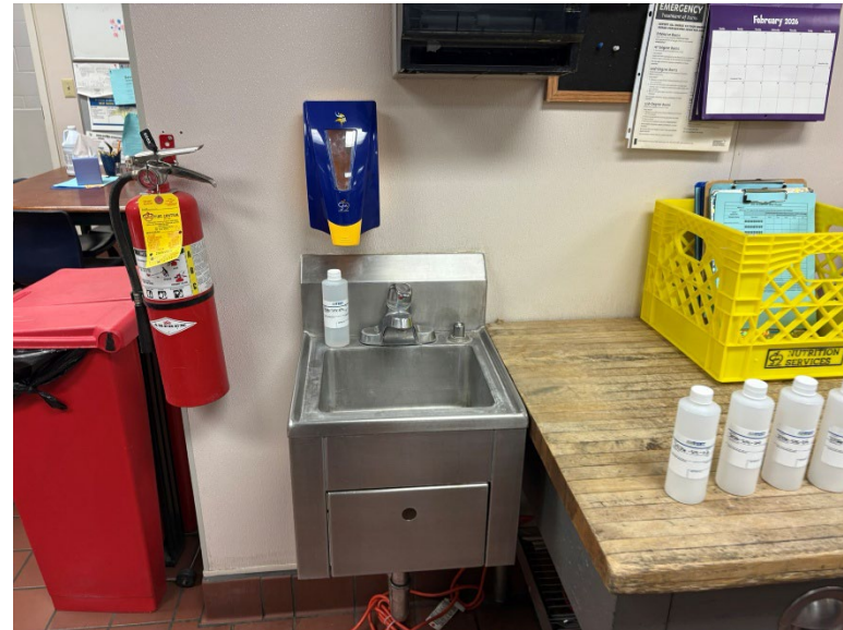
Kitchen South Handwash Tap – Sample 31126-SIS-02
