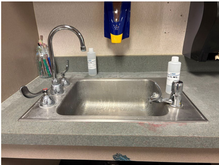
Room 301 Tap – Sample 31126-SIS-85 Room 301 Fountain – Sample 31126-SIS-86
