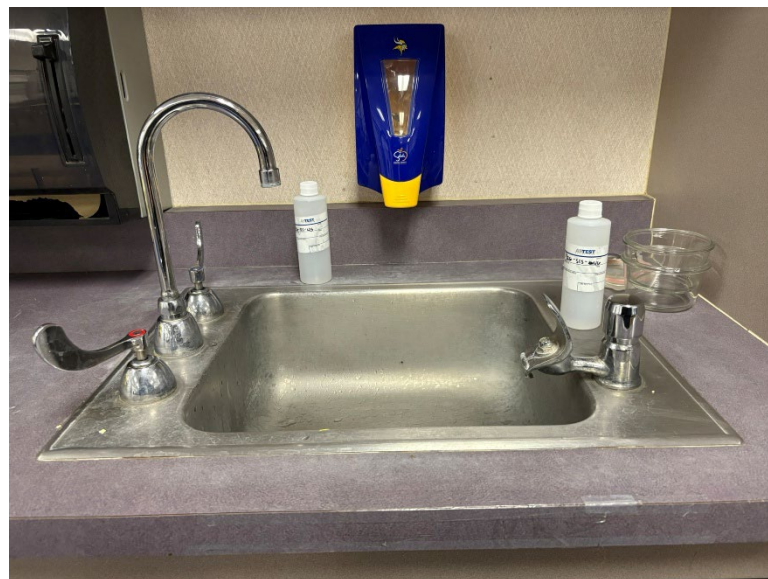
Room 112 Tap – Sample 31126-SIS-45 Room 112 Fountain – Sample 31126-SIS-46
