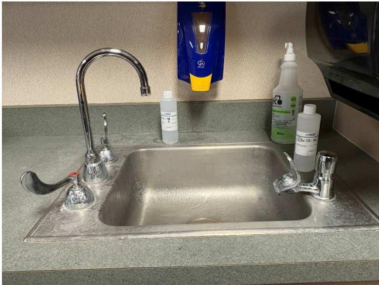
Room 303 Tap – Sample 31126-SIS-81 Room 303 Fountain – Sample 31126-SIS-82
