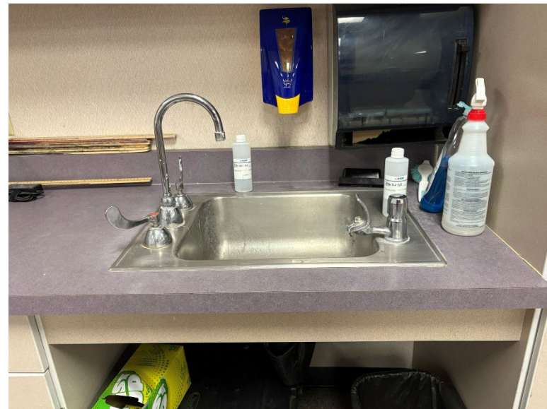
Room 107 Tap – Sample 31126-SIS-34 Room 107 Fountain – Sample 31126-SIS-35
