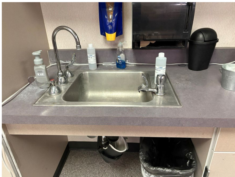
Room 109 Tap – Sample 31126-SIS-36 Room 109 Fountain – Sample 31126-SIS-37
