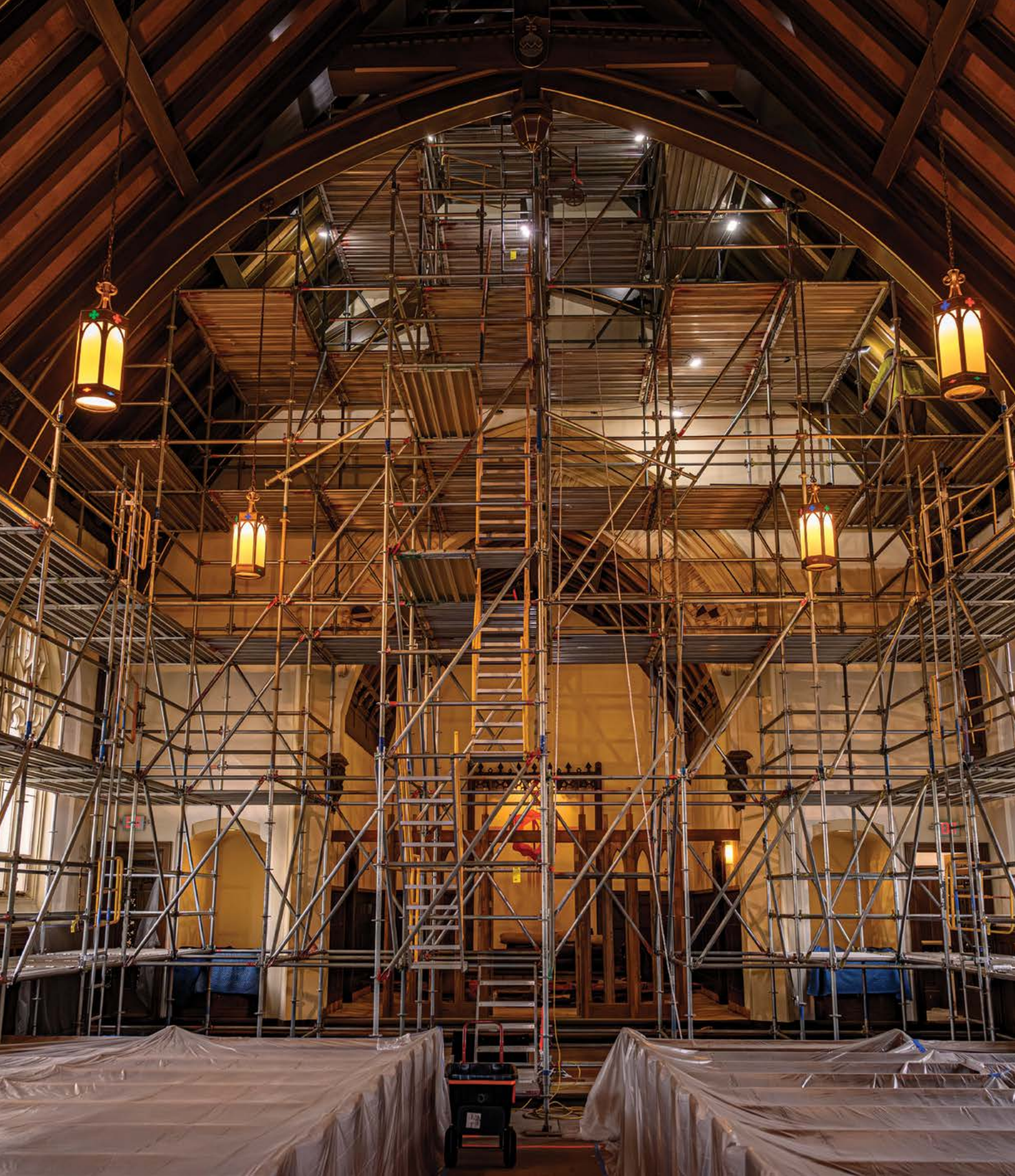
Our historic St. John the Evangelist Chapel is more beautiful than ever after undergoing significant repair work in 2025-2026. Important renovations included: replacement of select exterior roof tiles, plaster repair, painting, select
