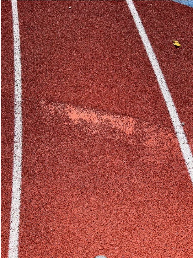
BH Track Damage (Dirt Bike) October 2023
