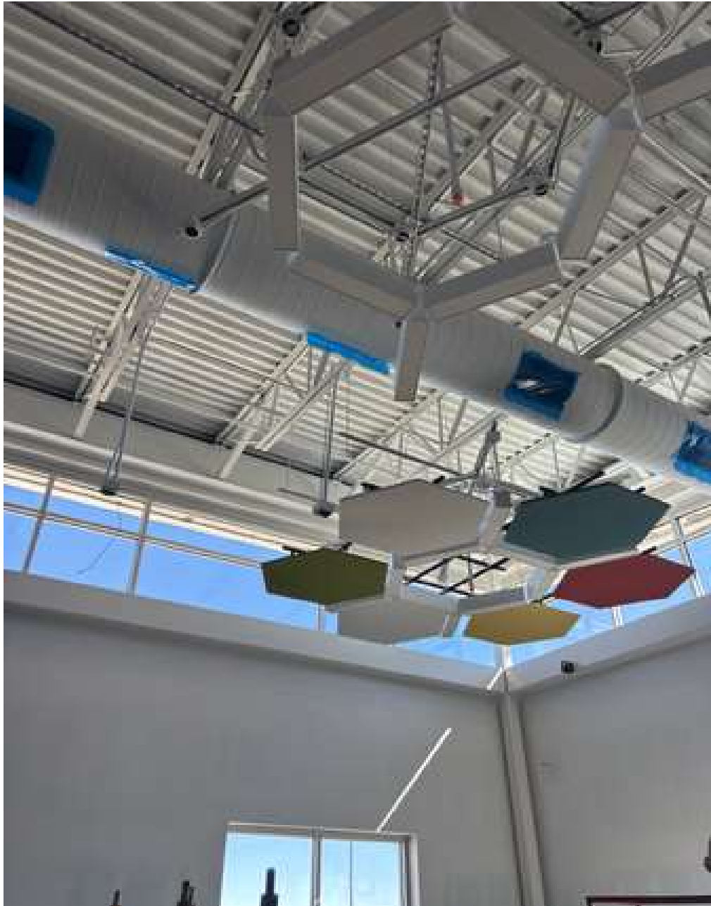
Media Center – Lighting
