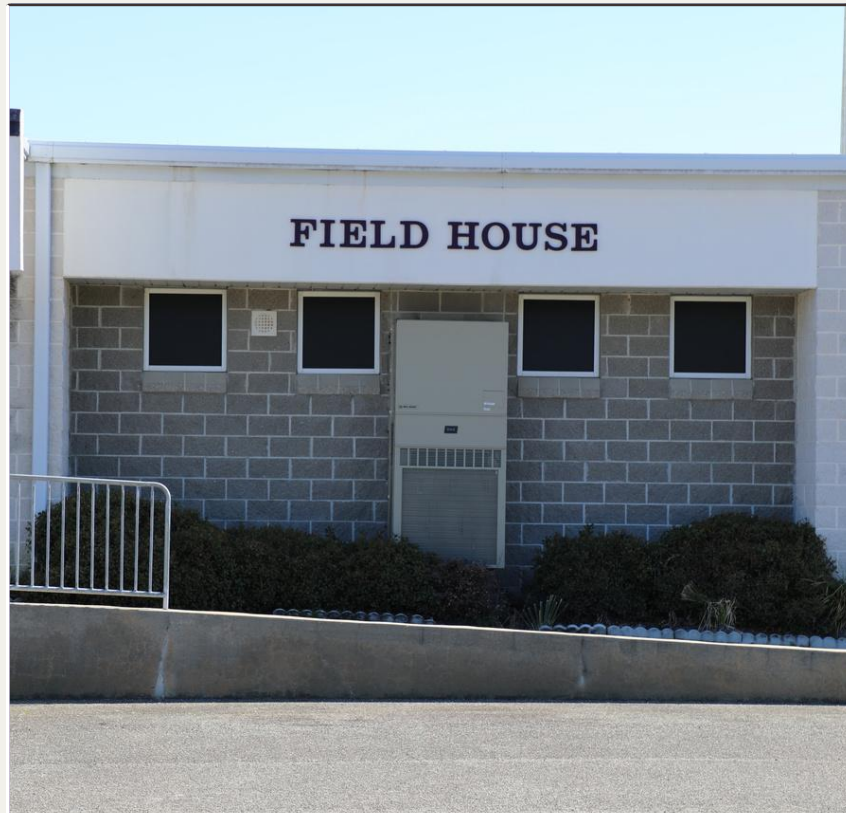
HVAC - Field House
