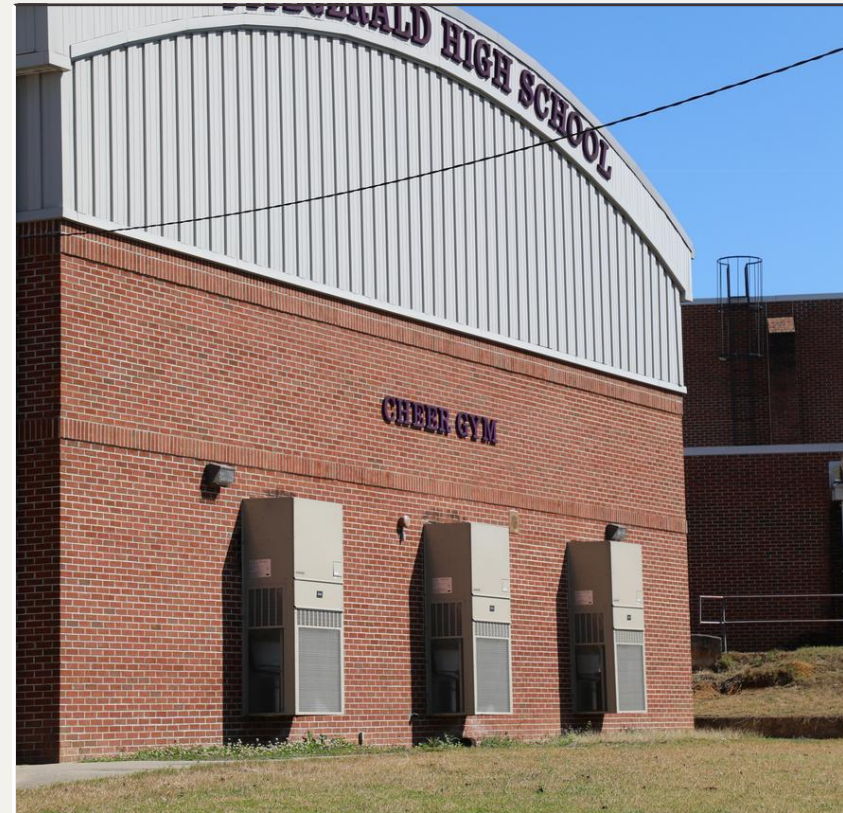
HVAC - Cheer Gym
