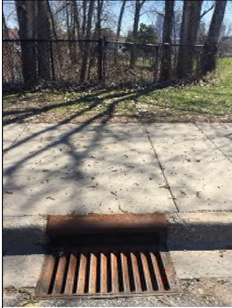
Final catch basin before pond – CB #5
