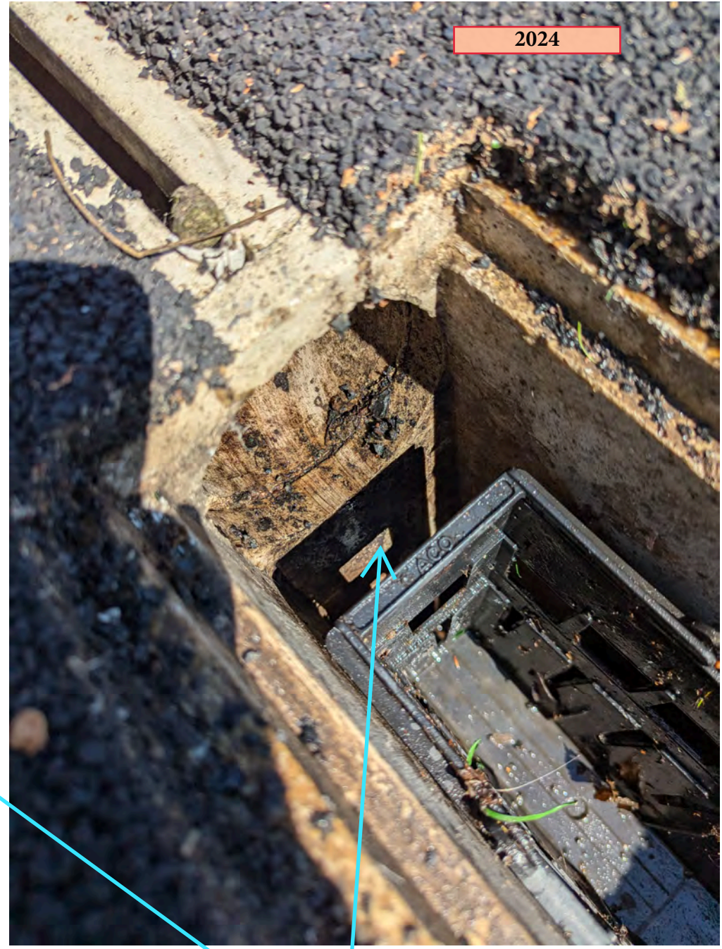
Note how basket sits on top of jutting PVC pipe, causing gaps and disconnection between channel and catch basin
