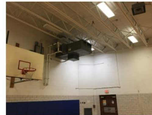
Picture 8: Typical Hot Water Air Handling Unit serving Gymnasium with Floor Mounted Return Register
