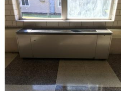
Picture 7: Classroom Unit Ventilator Serving Cafetorium
