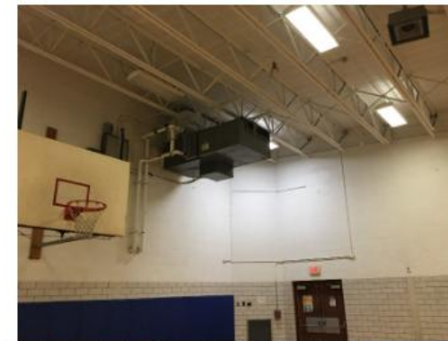
Picture 8: Typical Hot Water Air Handling Unit serving Gymnasium with Floor Mounted Return Register
