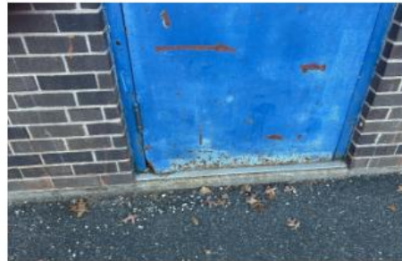
Typical Door Deterioration
