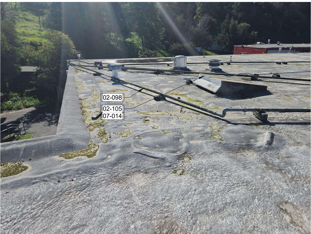
ROOF UNDULATIONS & BLISTERING
