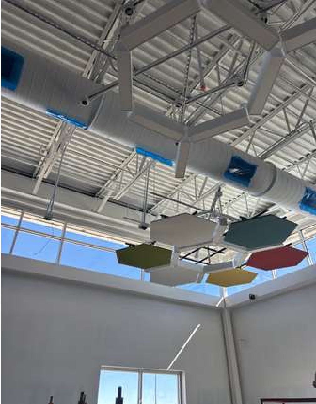
Media Center – Lighting
