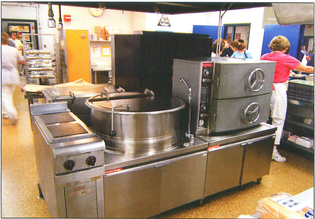
The cooking battery is outdated and needs replacement so that it can better serve the modern school lunch program. The kettle and steamer is difficult to use. New equipment can address ergonomics and reduce the risk for potential injury.
