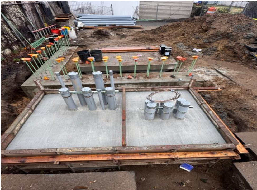
Hempstead IAQ – Paterson Transformer Pad
