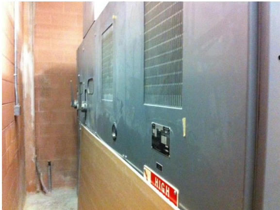
Figure 1 - Inadequate clearance space at Substation #1
