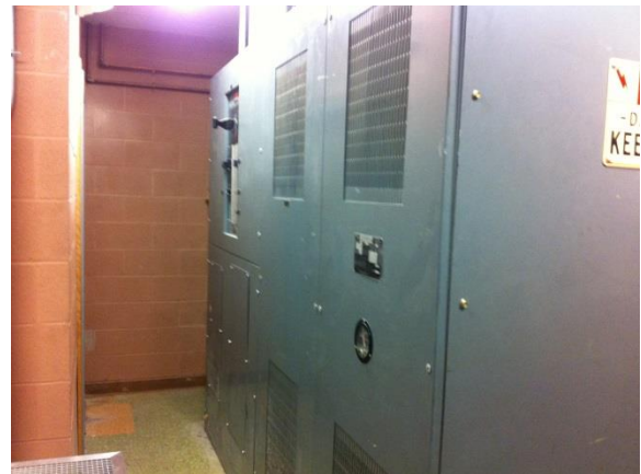
Figure 2 - Inadequate clearance space at Substation #2
