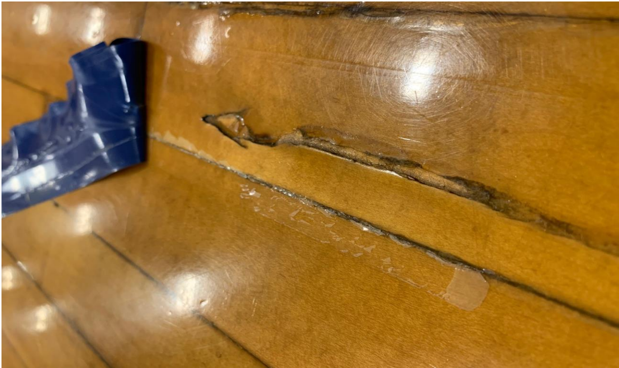
Crack in floor
