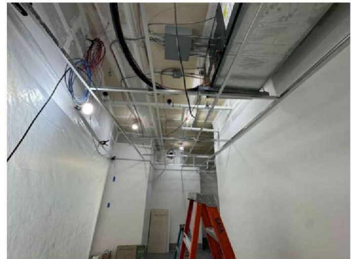
PR08 Overhead MEP & Ceiling Grid
