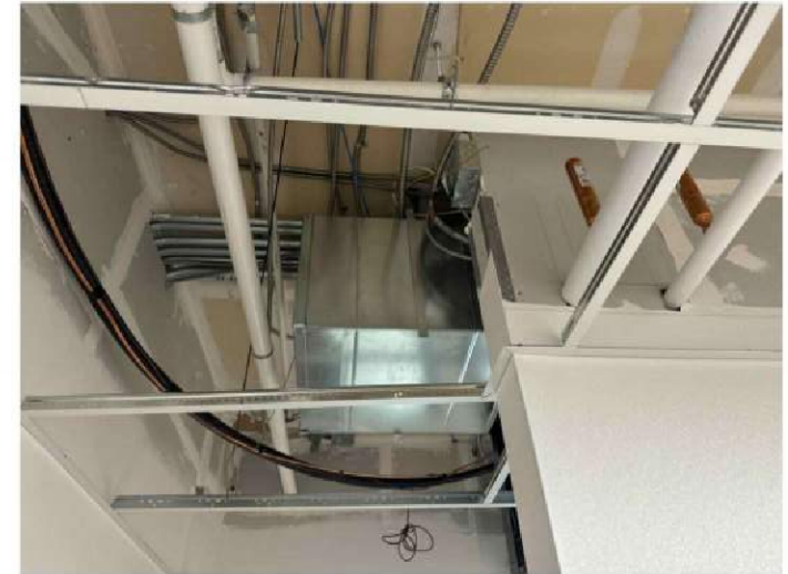
PR08 Overhead MEP in Kitchen
