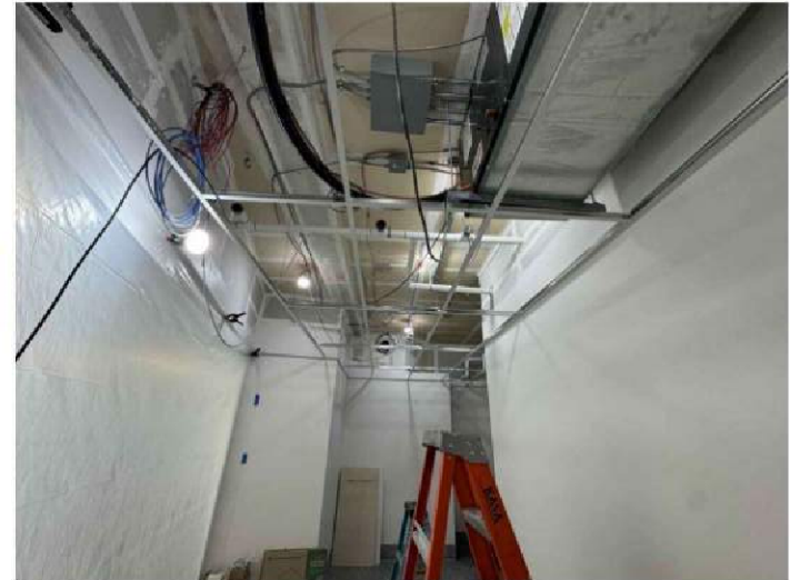
PR08 Overhead MEP & Ceiling Grid
