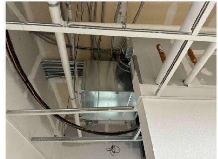
PR08 Overhead MEP in Kitchen
