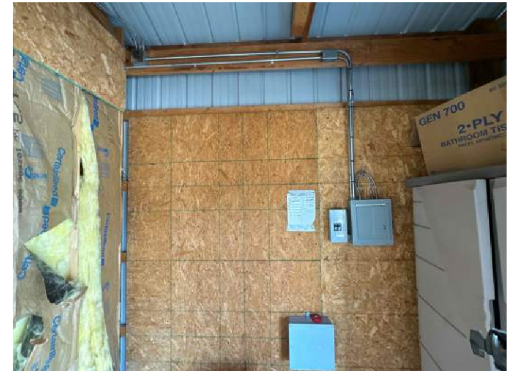
Concession Building Electrical
