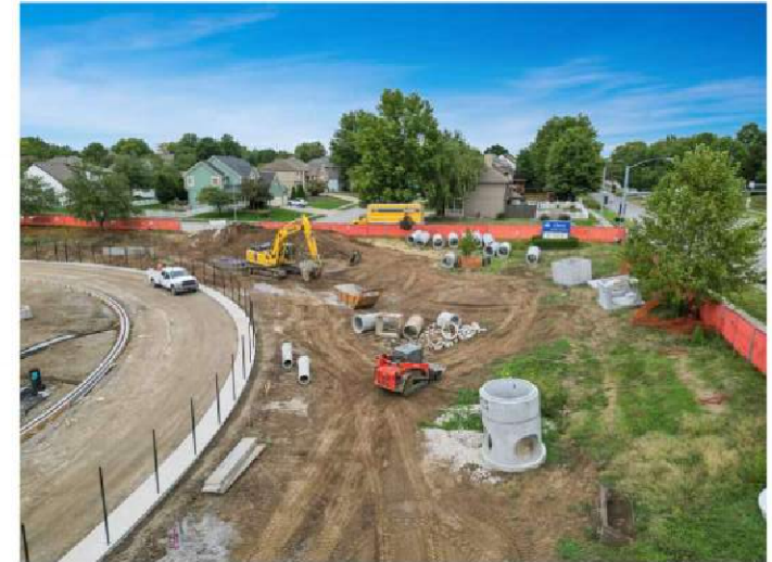
Public Utilities STM 1
