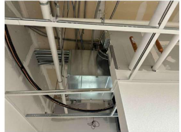
PR08 Overhead MEP in Kitchen
