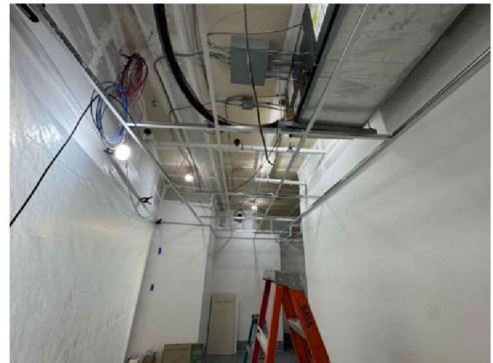
PR08 Overhead MEP & Ceiling Grid
