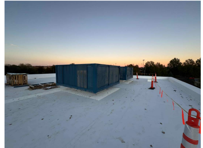
EPiC Elementary - RTU/Screens
