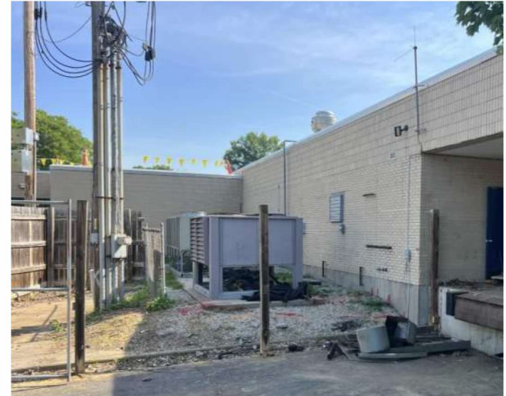
Alexander Doniphan - New Transformer Preparation
