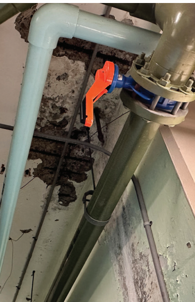
Basement ceiling and wall repair needed due to a pool leak.
