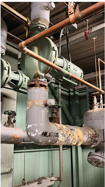
District-wide boiler room repairs and equipment replacement needs.
