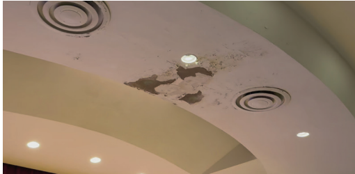
Auditorium ceiling repairs needed due to roof leak.
