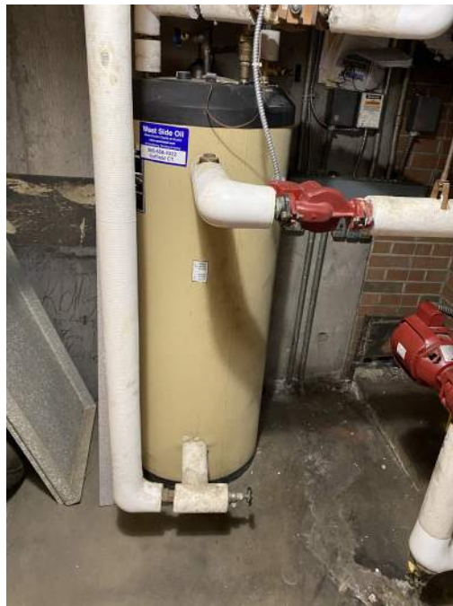
● D2. 23: Indirect Domestic Hot Water Heater
