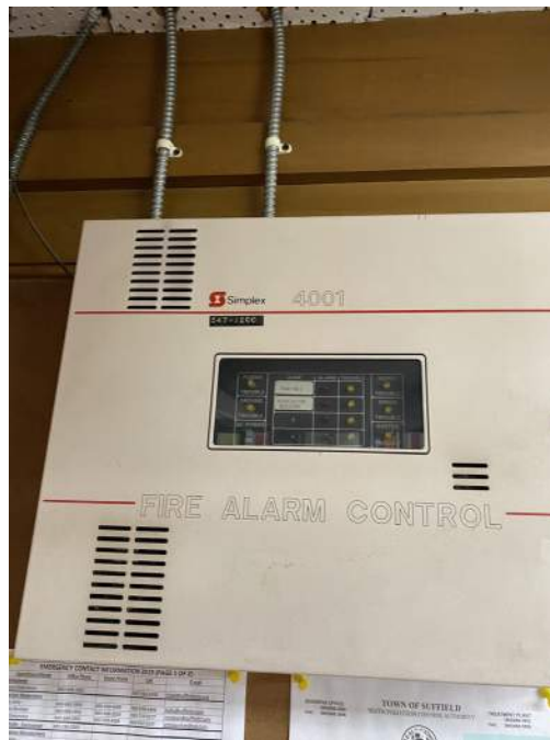
● D2. 16: Fire Alarm Control Panel
