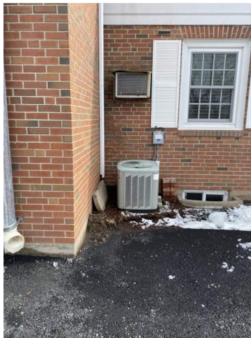
● D2. 8: Condensing Unit Serving FCU Provideing Cooling
