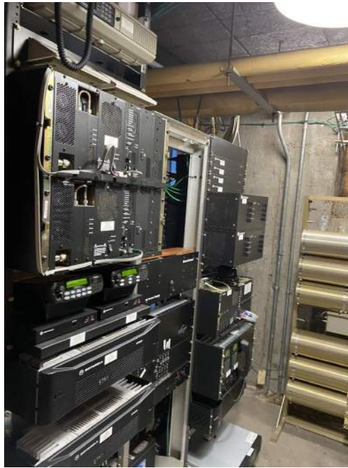
● D2. 37: Radio Equipment Rack
