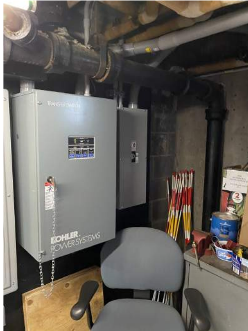
● D2. 3: Automatic Transfer Switch
