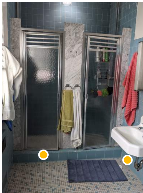
● D1. 12: Shower facilities are not wheel-chair accessible and sink does not have required pipe insulation to be considered ADA-compliant
