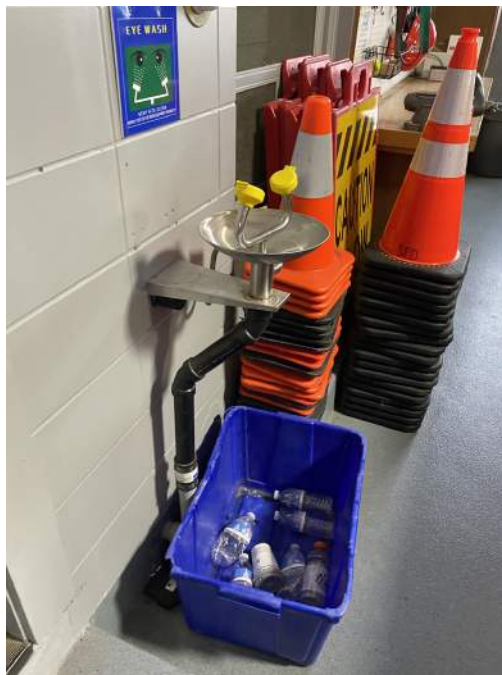
● D2. 14: Eyewash Station in Fair Condition
