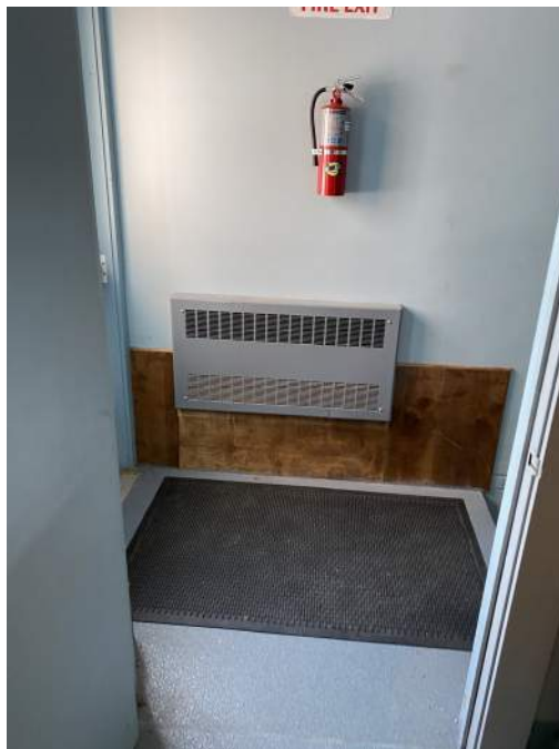
● D2. 18: Hot Water Wall Convactor Needs Replacing
