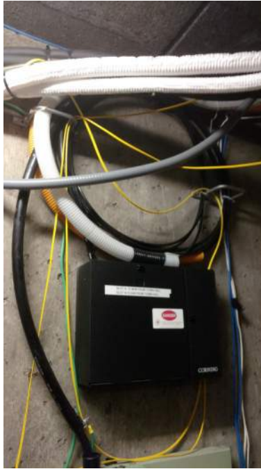
● D2. 15: Fiber Optic Service Equipment
