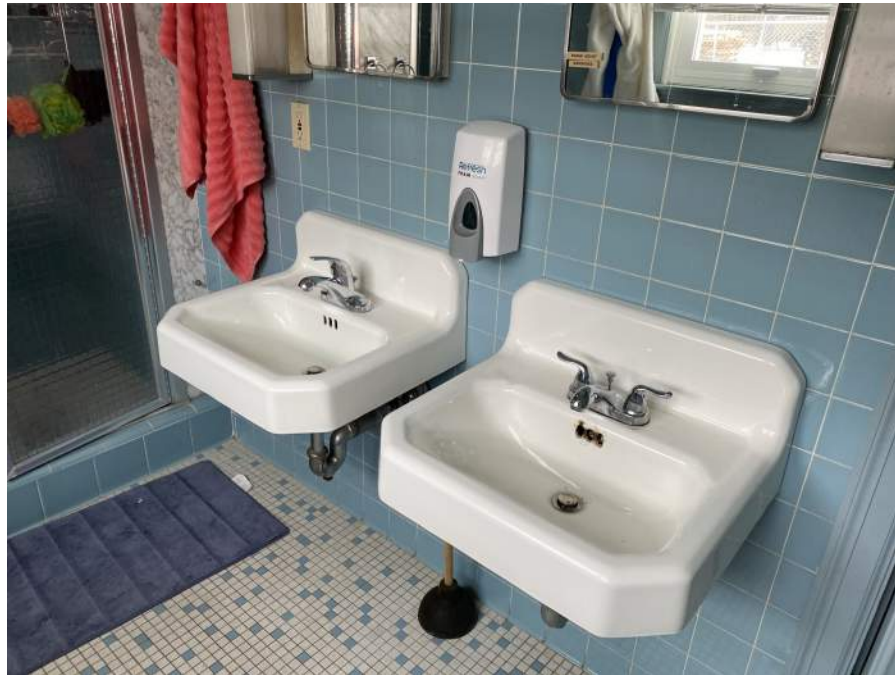
● D2. 35: Outdated Plumbing Fixtures
