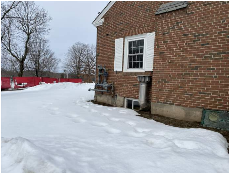
● D2. 29: Natural Gas Service
