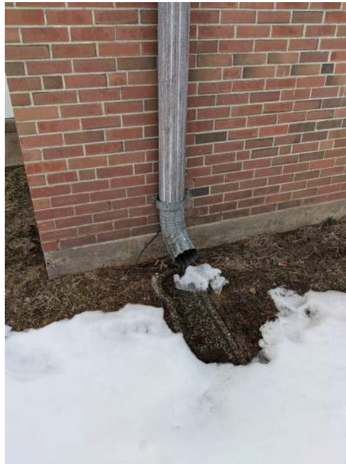
● D1. 7: Downspout splash block is under-sized, some soil erosion observed
