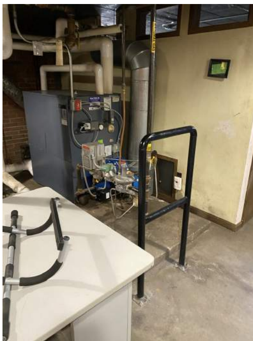
● D2. 28: Natural Gas Hot Water Boiler
