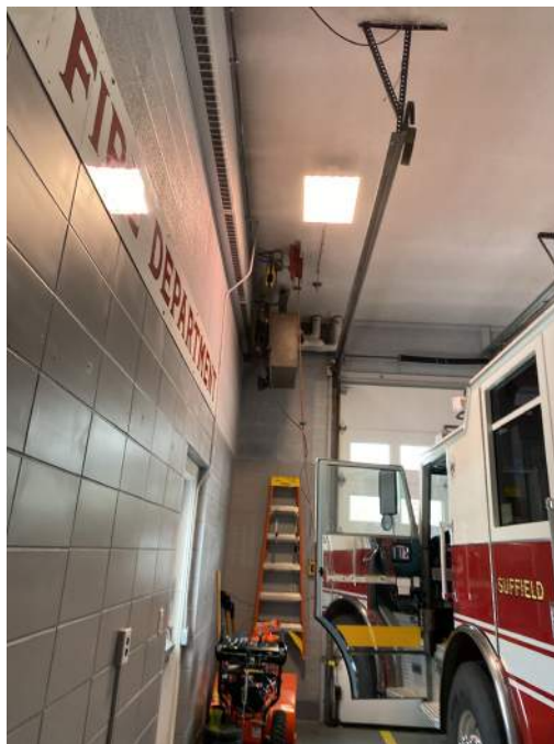
● D2. 2: App Bay Lighting - LED Fixtures
