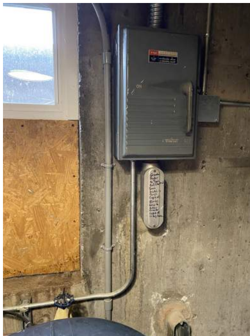
● D2. 30: Old Generator Feed to Town Hall
