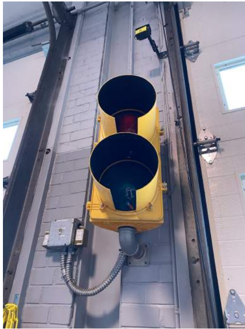
● D2. 25: Internal Traffic Control Light (Non-functional)
