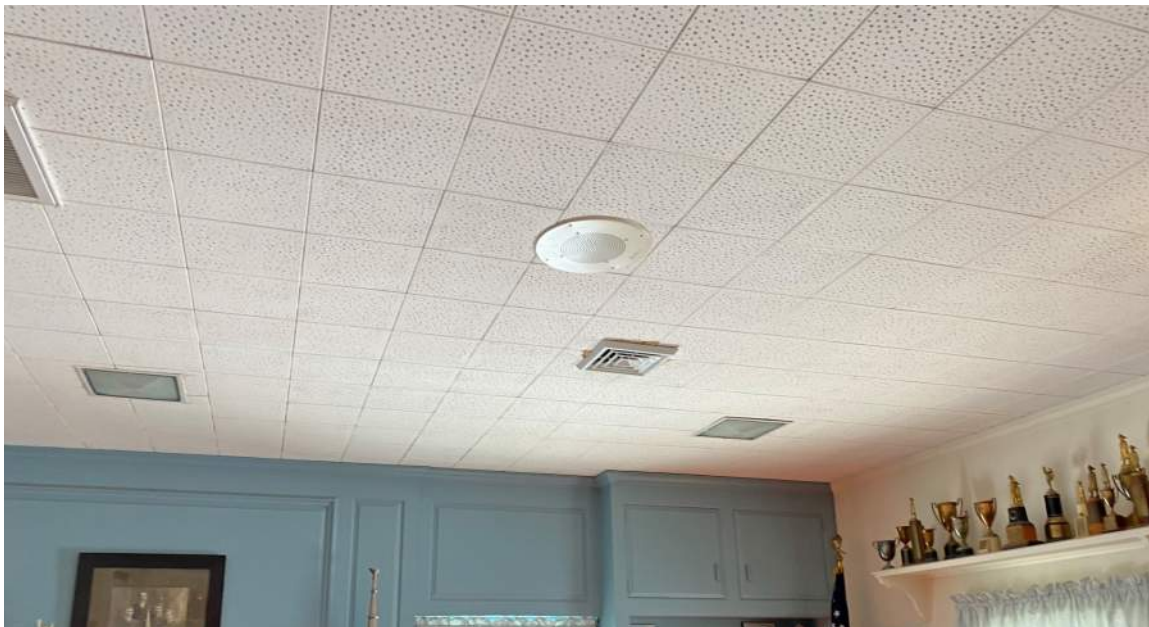
● D2. 34: Outdated Lighting
