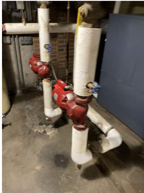
● D2. 19: Hydronic Hot Water Pumps
