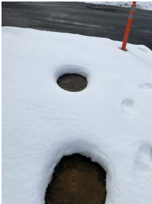
● D2. 27: Municipal Sewer Service Access
