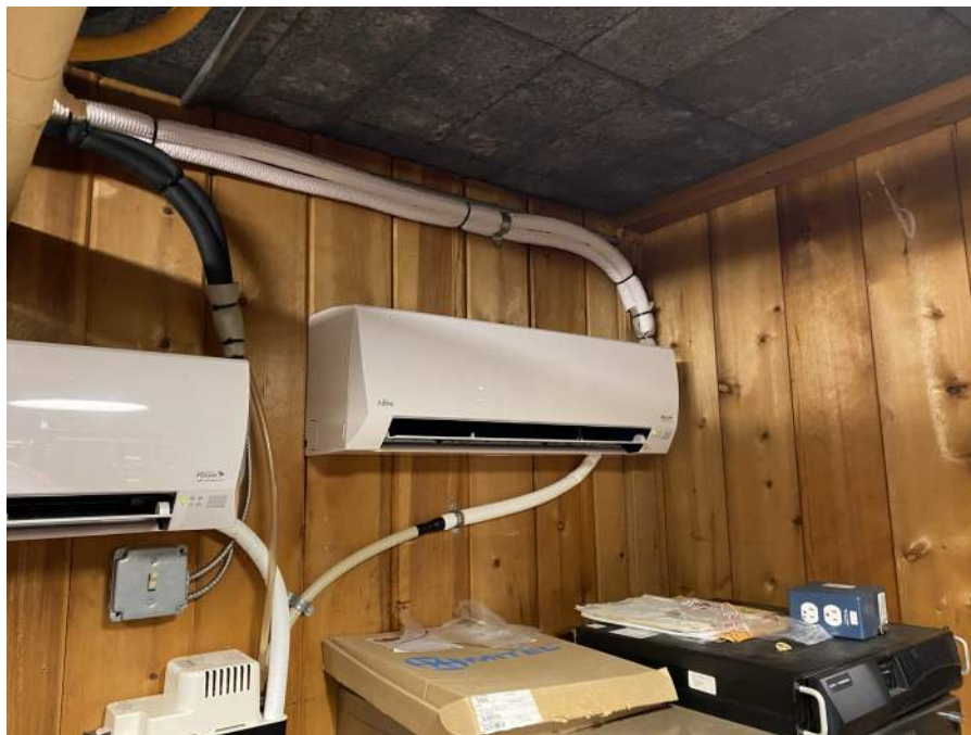
● D2. 22: IT Room Split AC Units
