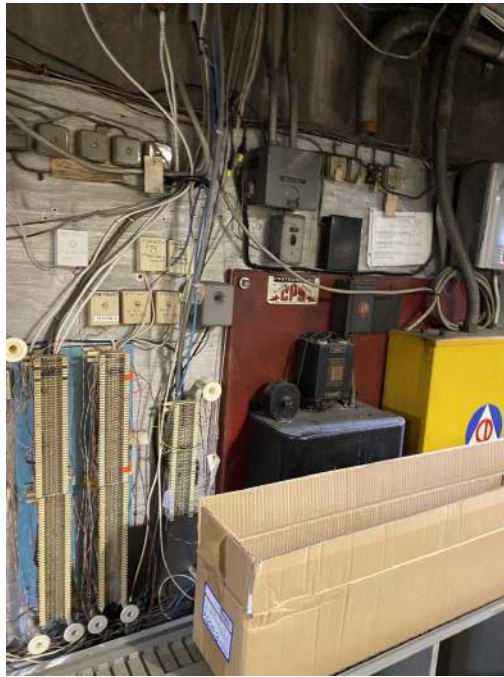
● D2. 33: Outdated Communication Infrastructure
