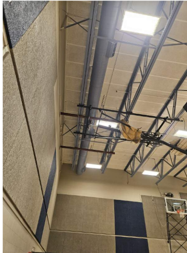
DMS - Wrestling Mat Hoist Support Steel
