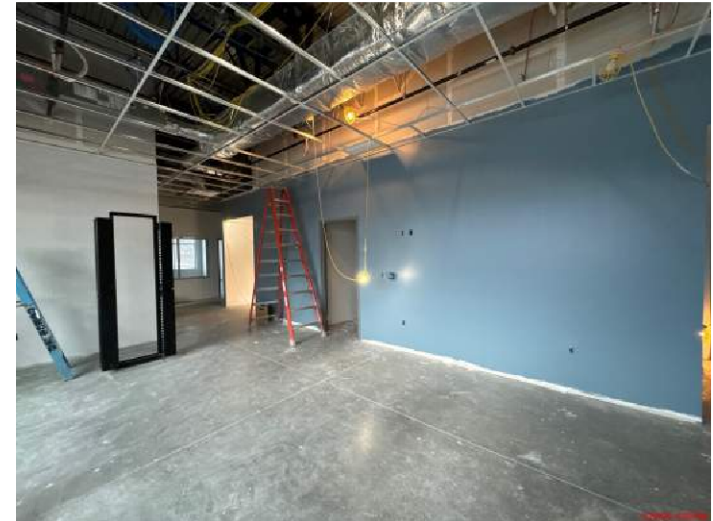
Workstation A105 Area
