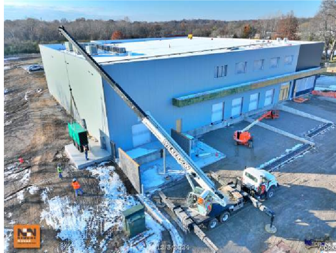
East Lot/Generator Set
