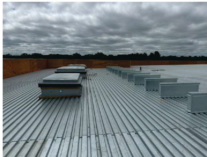
RTU and Condensing Unit Curbs
