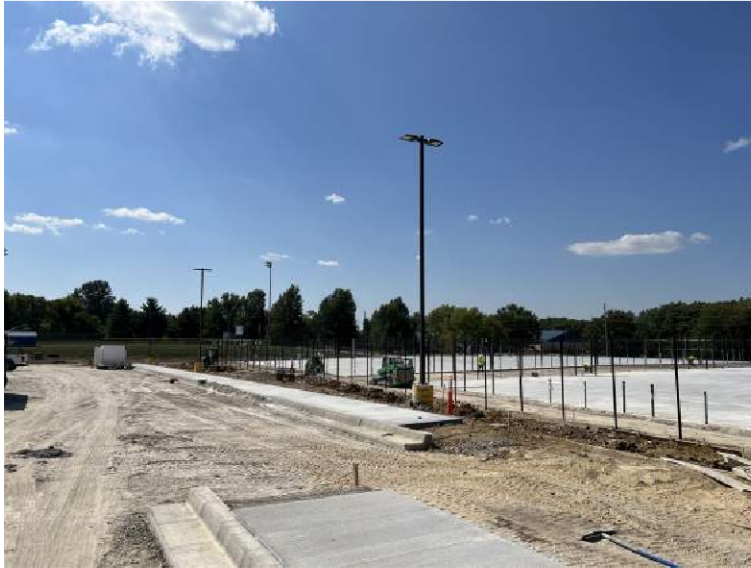
New Light Poles Looking East over Complex
