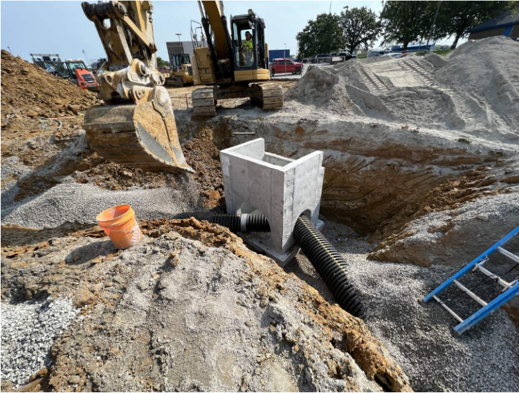
Site Storm Boxes / Drainage
