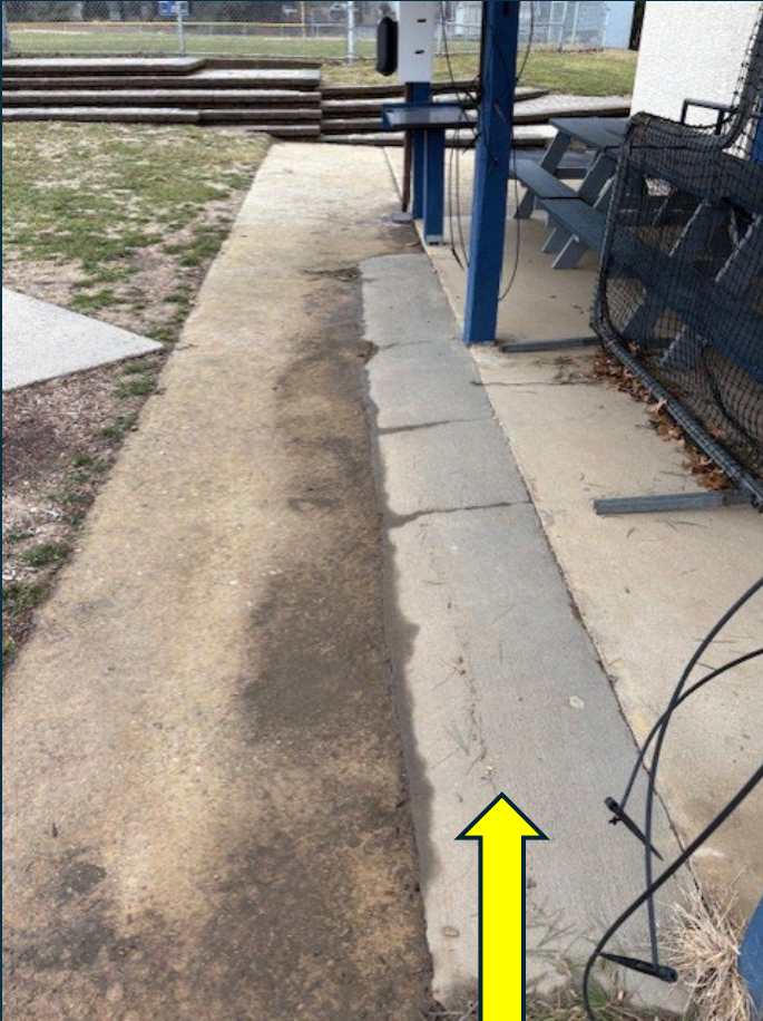
Settling has led to a need for patched "ramps"
