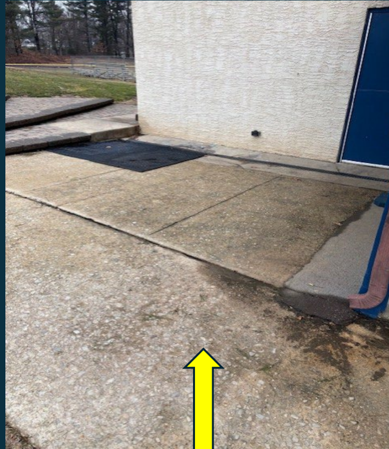
Erosion has led to exposed underlayment
