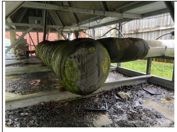
Photo #18. View of assumed ACBM TSI piping below west exterior HVAC equipment.
