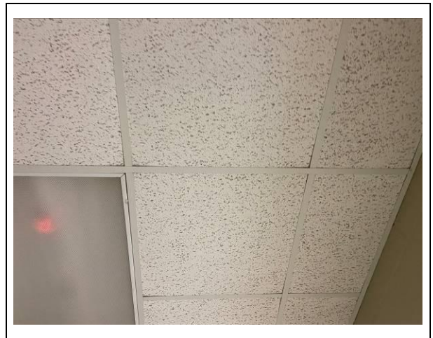
Photo #40. View of assumed ACBM 2'X2' white ceiling tile with pinholes in the gym.
