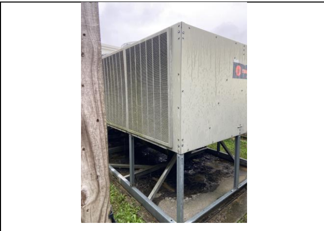
Photo #17. View of western exterior HVAC equipment with assumed ACBM TSI piping below.
