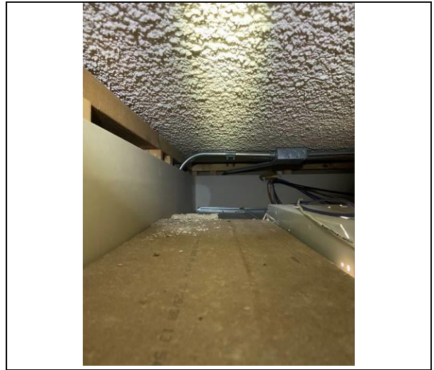
Photo #20. View of assumed ACBM white spray applied fireproofing located above ceiling tile in original bldg. & 1 st addition.
