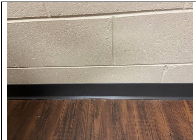
Photo #29. View of assumed ACBM gray cove base in special education room #4.
