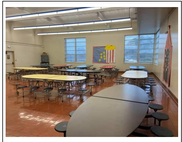
Photo #4. Typical assumed ACBM observed in the cafeteria of the original bldg.
