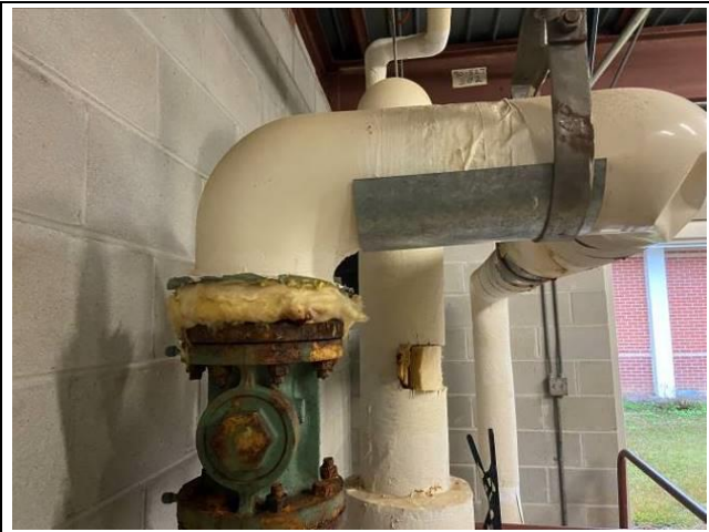
Photo #15. View of assumed white covered yellow straight run/elbow insulation in exterior HVAC room.
