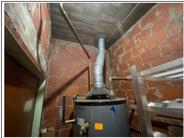
Photo #9. View of assumed brick and grout in water heater closet in original bldg.
