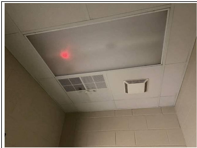
Photo #39. View of assumed ACBM 2'X2' white smooth ceiling tile in the gym.
