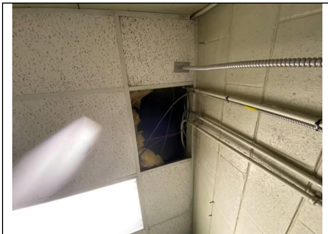
Photo #41. View of assumed ACBM yellow insulation above the ceiling tile in the gym.
