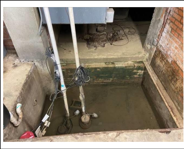
Photo #13. View of HVAC equipment near crawl space in exterior HVAC room.
