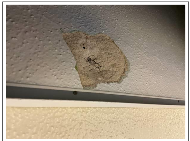
Photo #42. View of typical negative ACBM plaster found throughout the original school.
