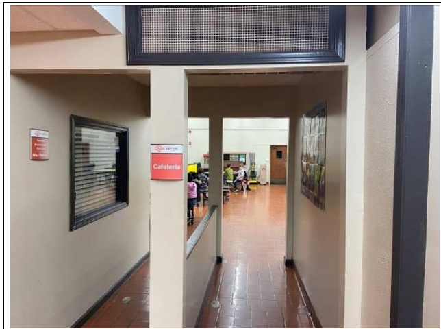
Photo #3. Typical assumed ACBM sheetrock observed by the cafeteria.
