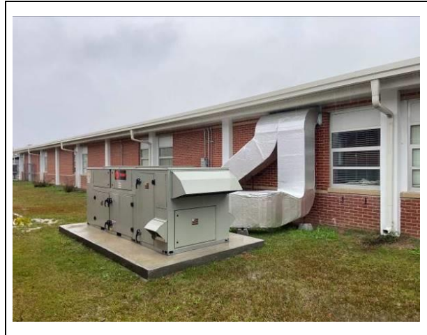
Photo #16. View of assumed ACBM silver duct along western exterior of school.
