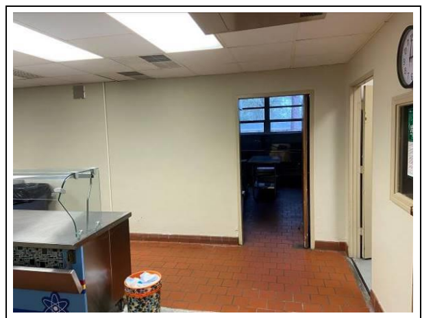
Photo #6. View of assumed ACBM materials in the kitchen of the original bldg.
