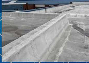
Tear off all wall flashing. Mechanically attach 1/2" HD ISO cover board to all parapet walls
