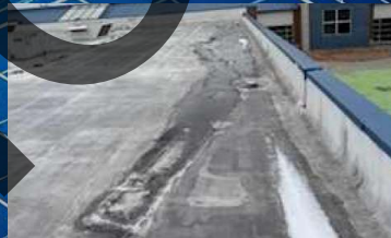
Area is wet. Replace Everything
