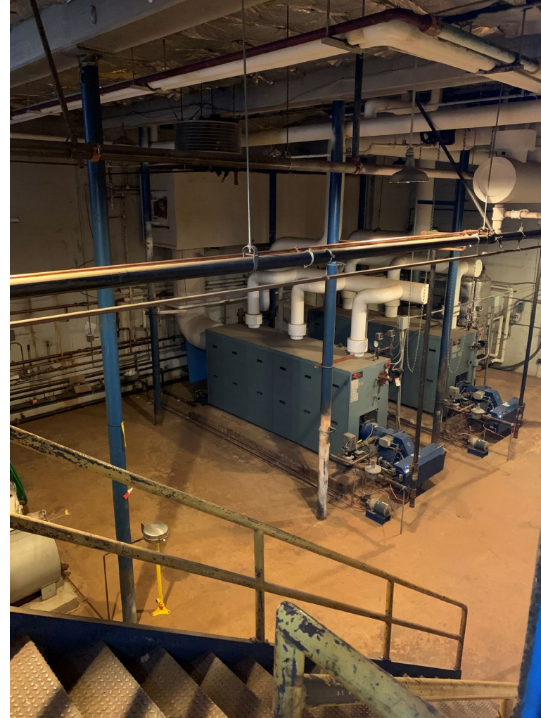
Outdated, inefficient boilers
