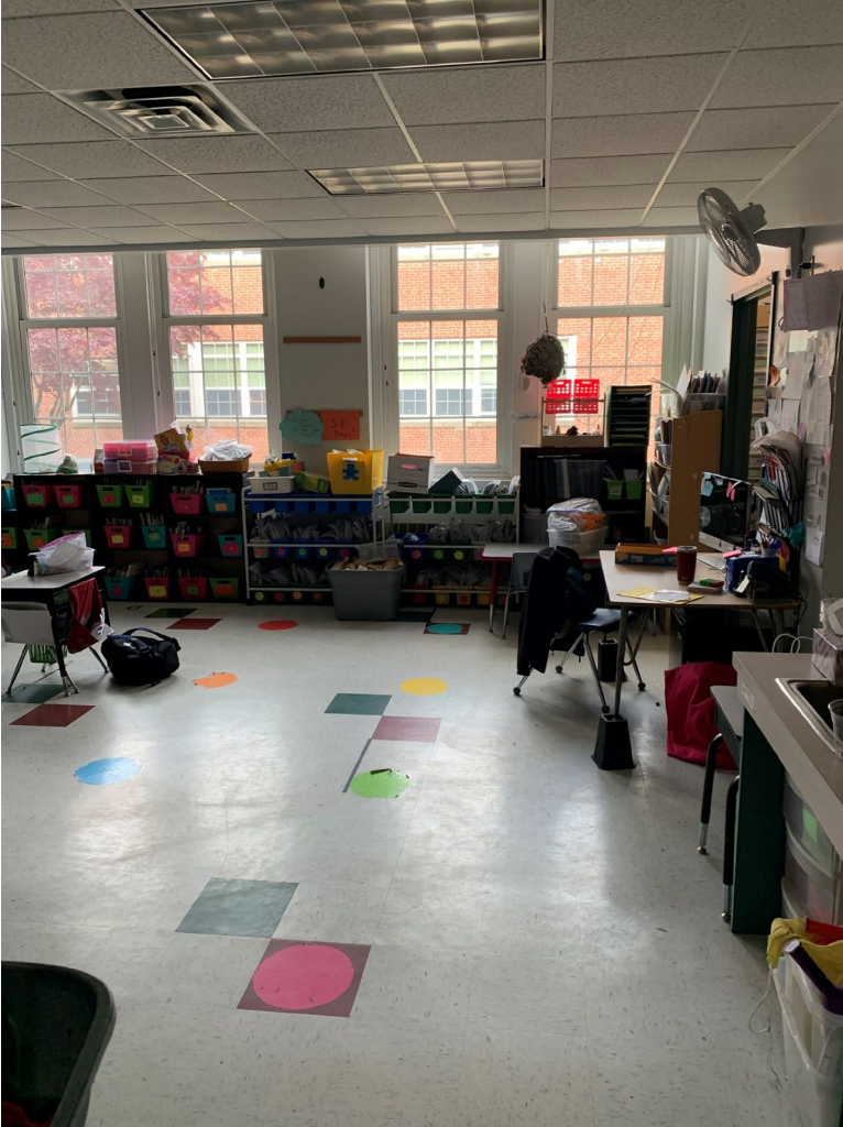
Classroom (Not air conditioned, lacking sufficient storage)
